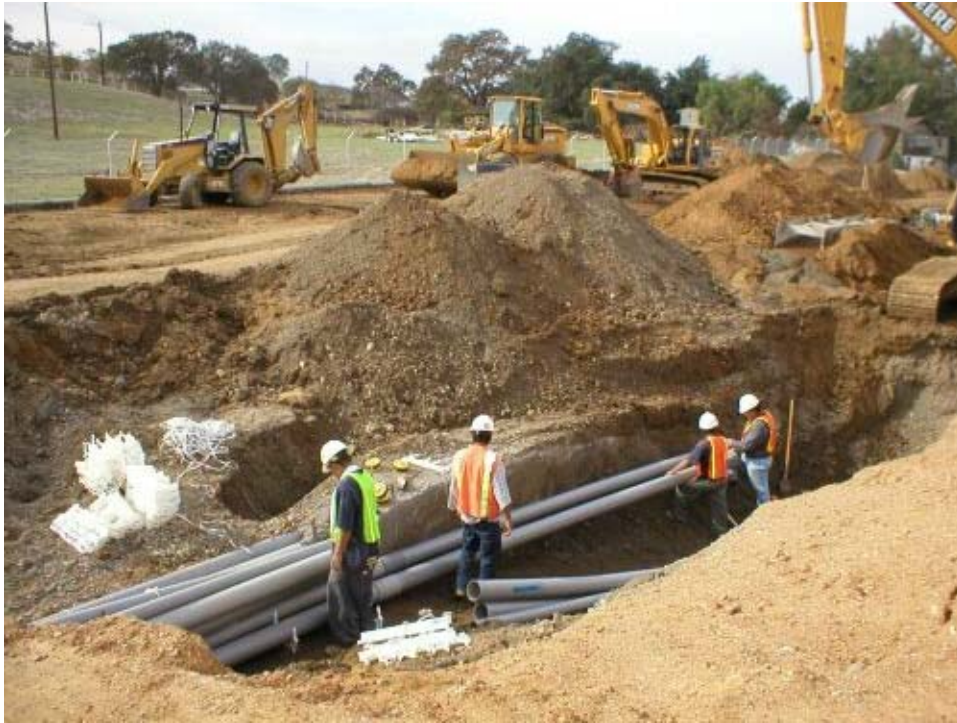
Figure 1 Deep trench and conduit installation around a storm drain within New Vineyard Road.
