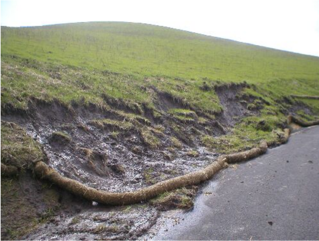
Figure 1 – Additional slumping in the road cut above Road 6, March 6, 2006.
