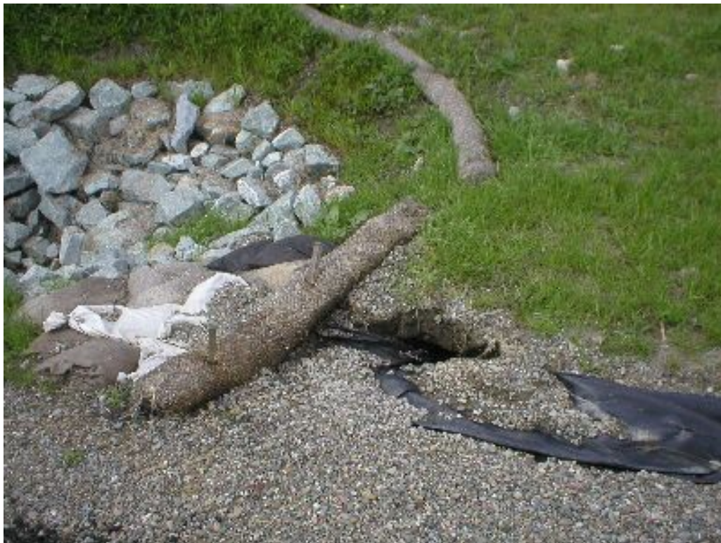
Figure 4 – Undercutting of a culvert inlet along Moller Road, March 6, 2006.
