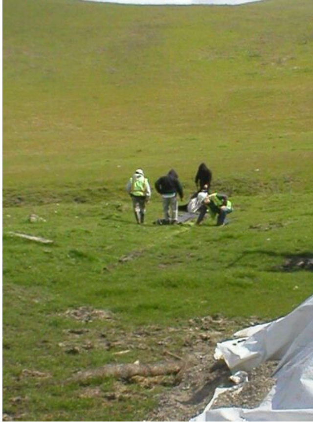
Figure 1 – North Valley crews escorted by a biologist removing damaged sediment fence, March 15, 2006.
