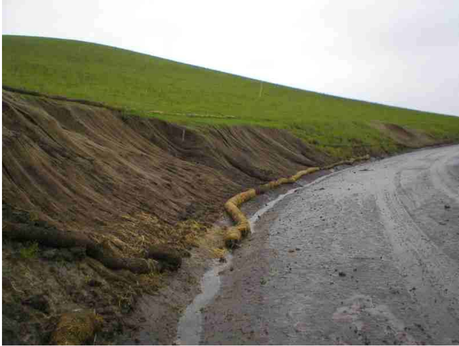
Figure 1 – NVC crews removed slumped soils and re-installed jute netting and wattles over the Road 6 slump area, April 12, 2006.
