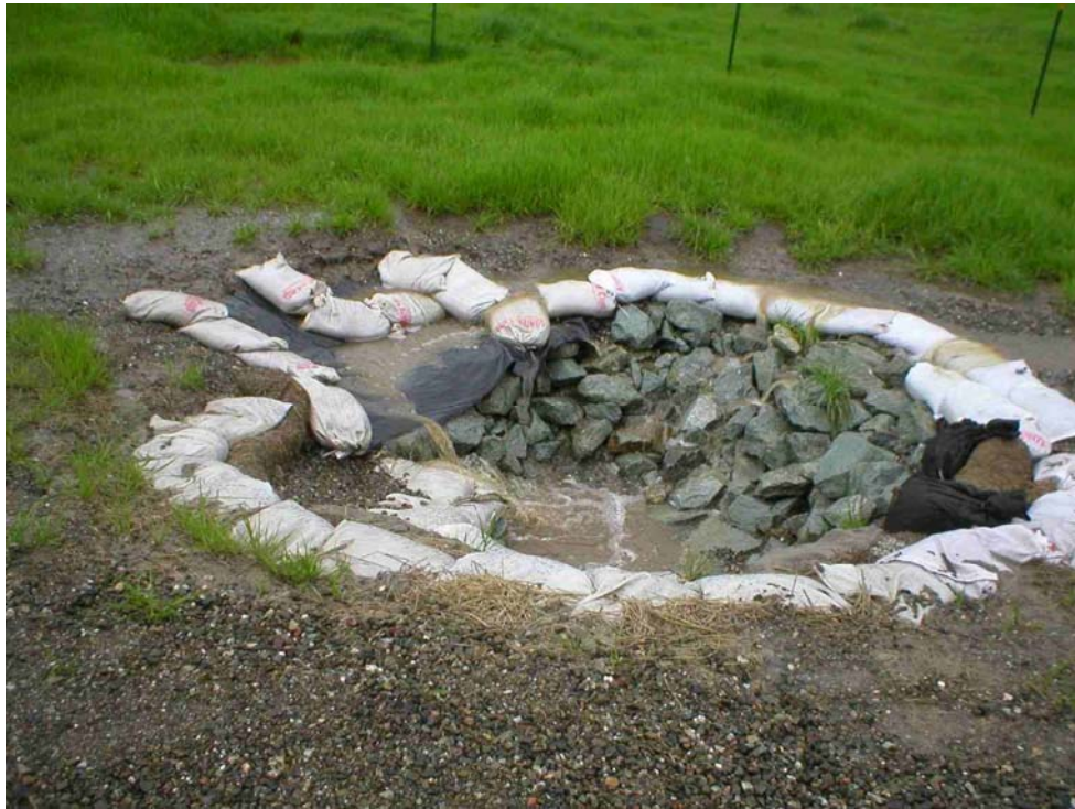
Figure 3 – Storm water flow into a culvert along Moller Road, April 10, 2006.
