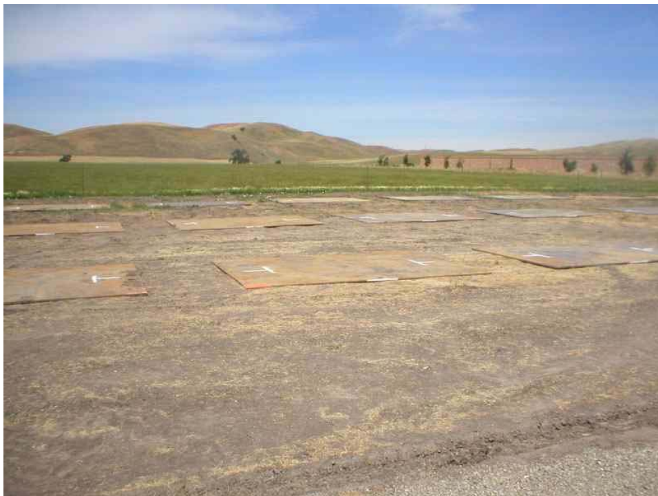
Figure 2 – Steel plates laid for transmission spool storage at the Wilson yard, June 2, 2006
