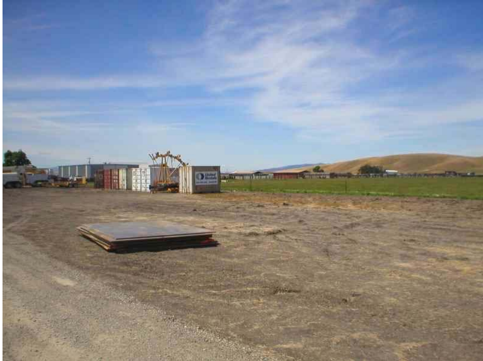
Figure 1 – Wilson yard, June 2, 2006. Note the equipment for the transmission line pulling activities.
