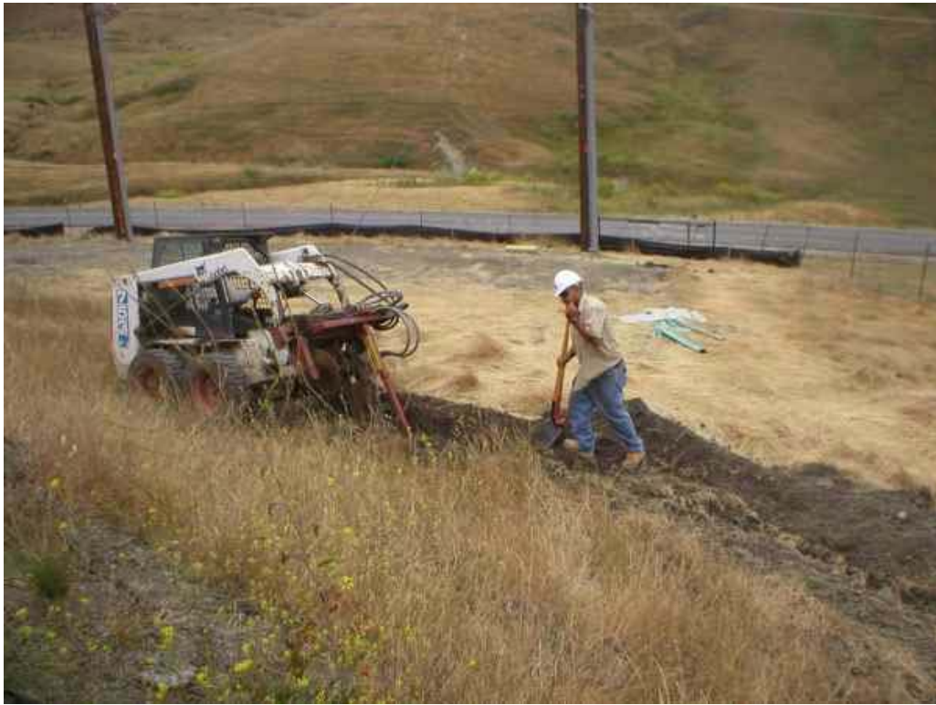
Figure 3 – Vitale and Sons trenching around the North Dublin Substation for installation of the irrigation line. June 13, 2006
