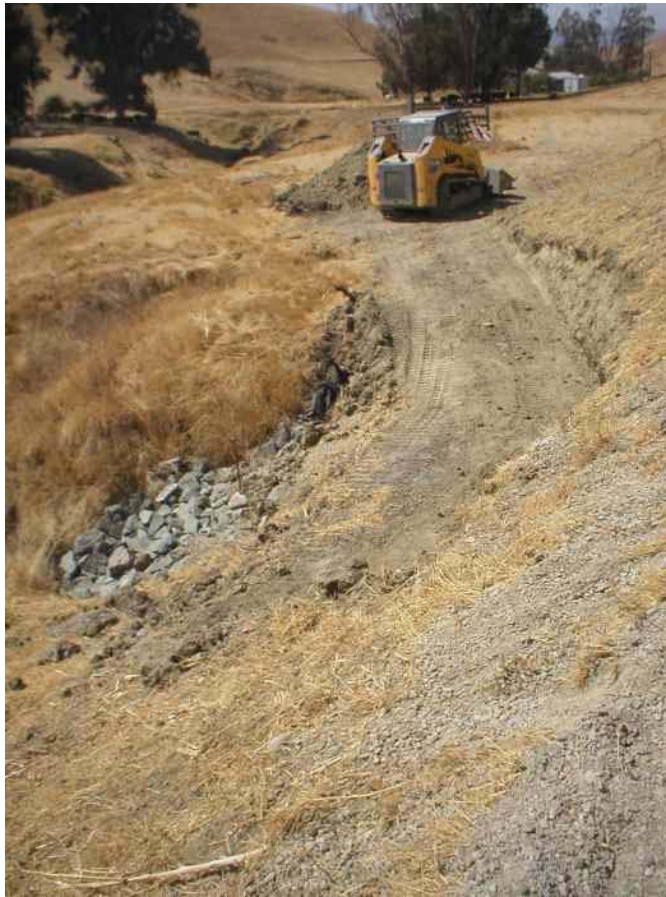
Figure 4 – Side slope stabilization and culvert work in an eroded area adjacent to Moller Road, August 18, 2006.
