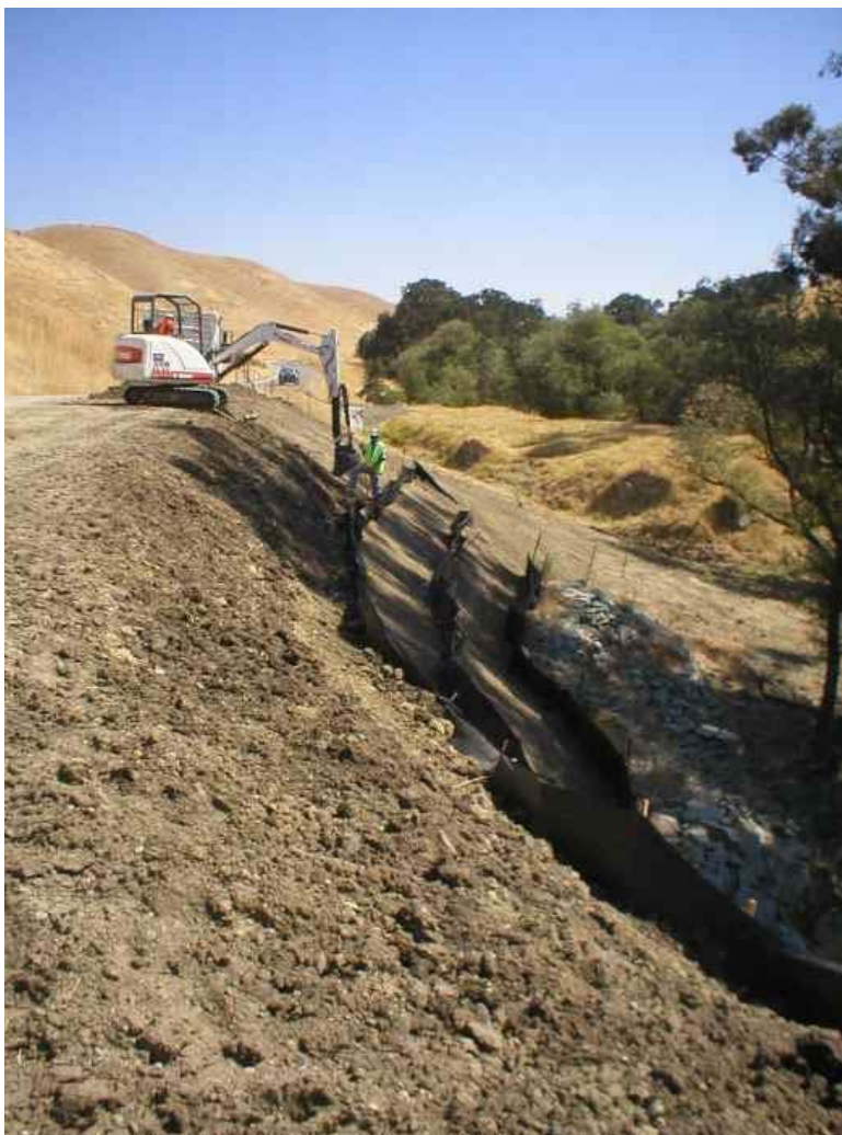
Figure 1 – NVC crews conducting bank and slope stabilization work near Tassajara Creek, August 18, 2006.
