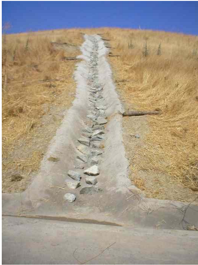
Figure 3 – V-ditch along a slope at Moller Road. Note the new concrete lining and imbedded rocks, August 18, 2006.
