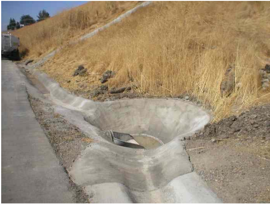
Figure 2 – Along Moller Road, eroded culverts were set in concrete. Rocks will later be replaced on the inlets and outlets, August 10, 2006.
