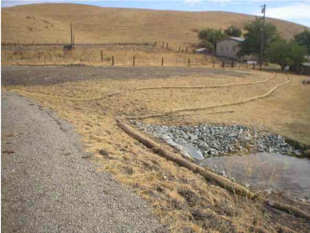
Figure 1 – Turnaround area. Note that the wattles have been installed to protect Cayetano Creek, October 4, 2006.
