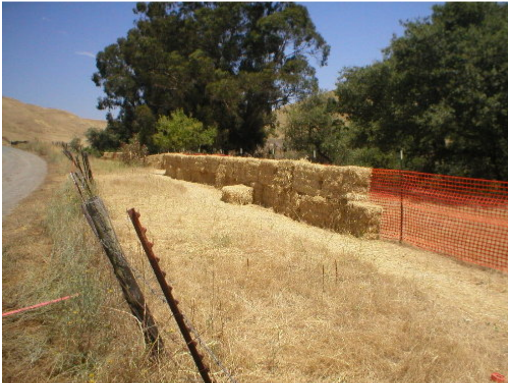
Figure 3 – Barn owl exclusion wall constructed along the Moller Ranch Road, Phase Three, July 15 th .
