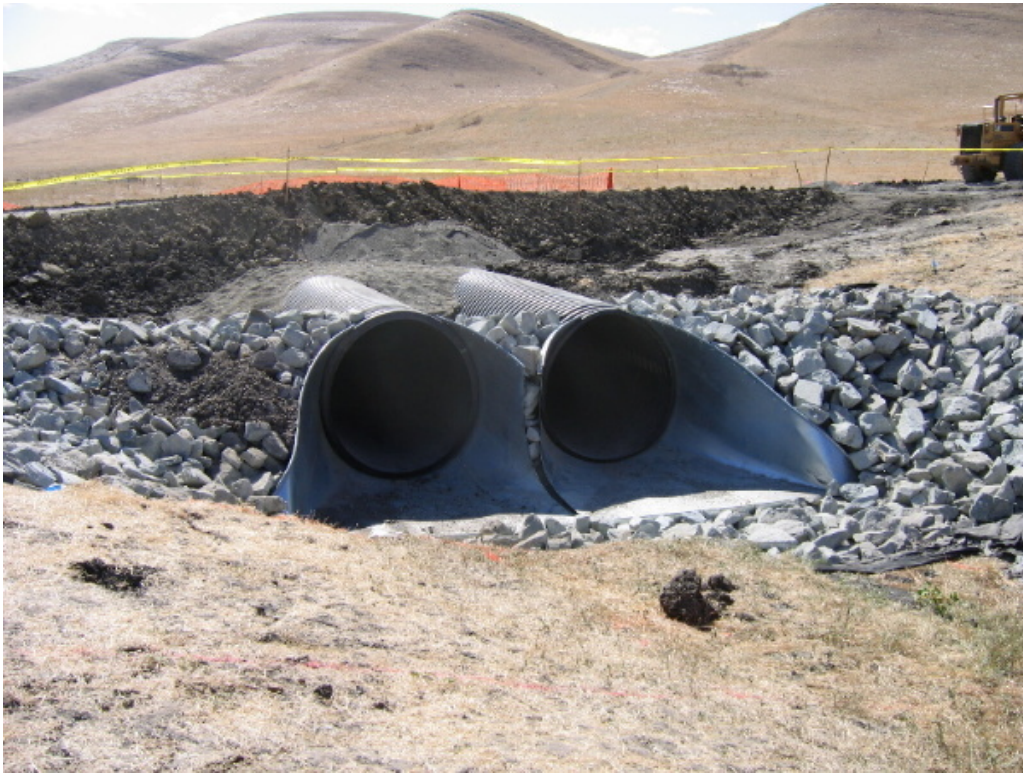
Figure 3 – Culvert installation at the crossing in Figure 2 was installed on September 24 th and 25 th .
