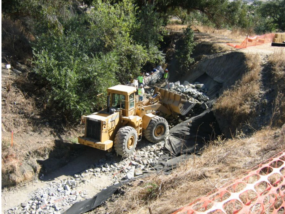
Figure 1 – Bank stabilization area within Tassajara Creek, October 11, 2005.
