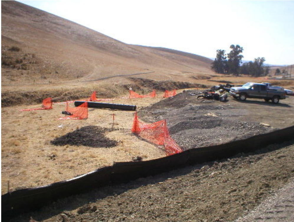
Figure 1 – Staging areas next to the Substation along Moller Ranch Road. Erosion controls need to be installed around spoils piles.
