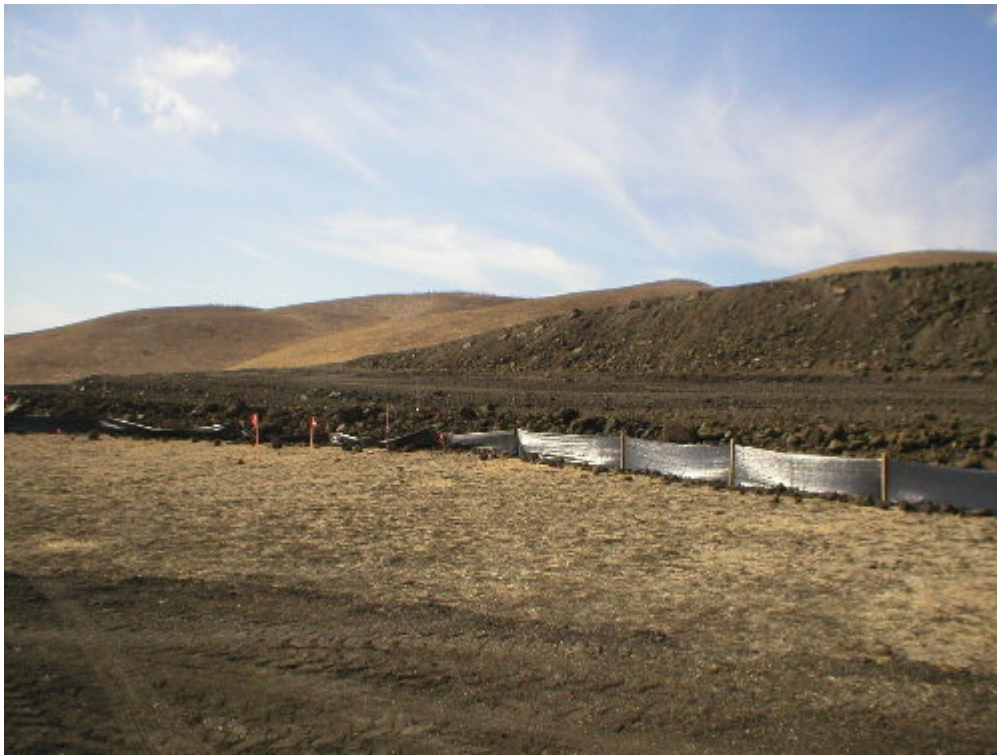
Figure 2 – Sediment fencing in need of repair next to the substation.
