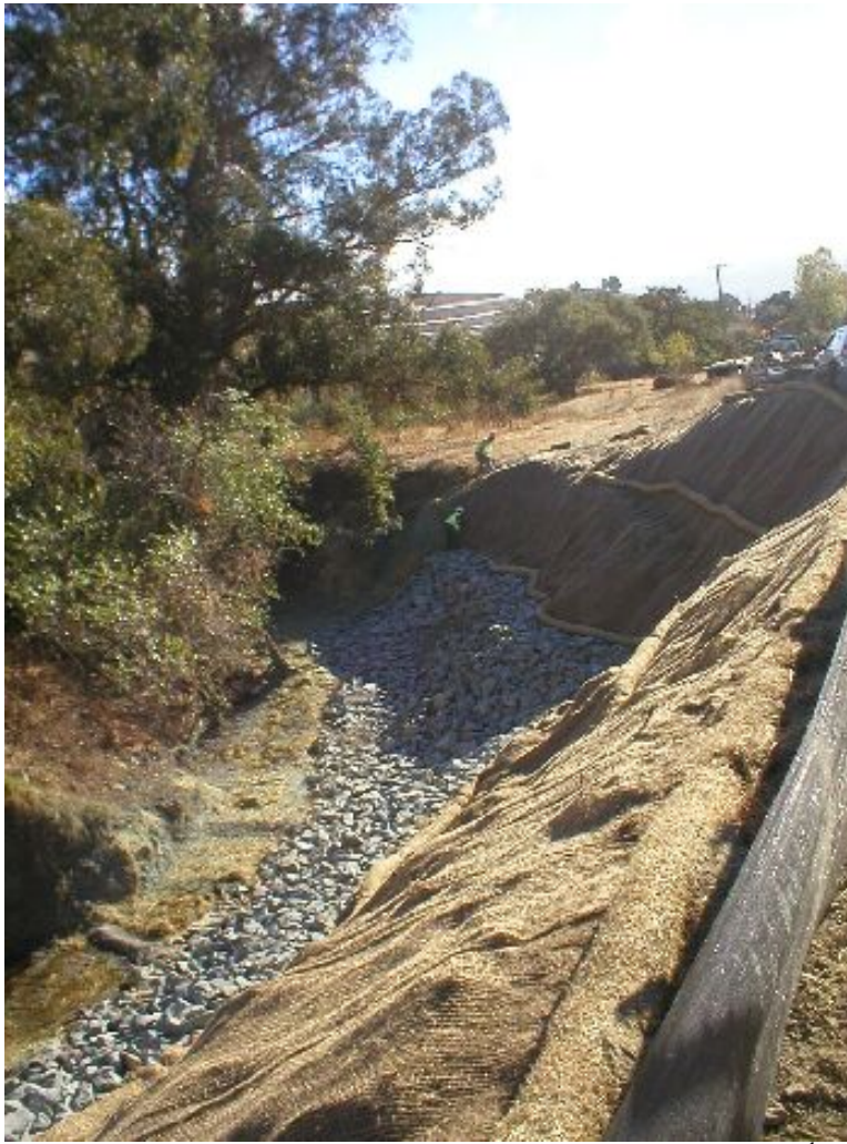
Figure 6 – Bank stabilization work in Tassajara Creek - November 4 th . Note the complete erosion controls.
