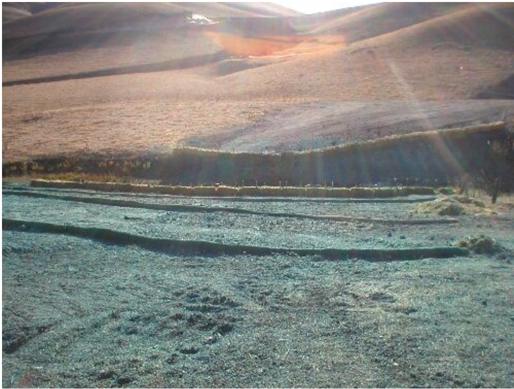
Figure 3 – Long slope over Cayetano Creek has installed BMPs for erosion prevention and sediment control.
