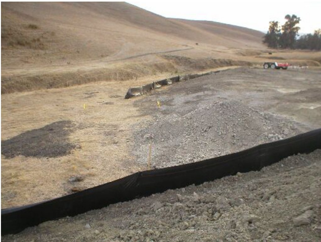
Figure 4 – Inadequate erosion controls around graded areas and a spoils pile located in a staging area adjacent to Tassajara Creek - November 1 st .
