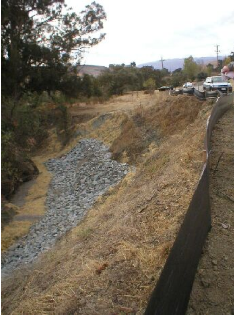
Figure 5 – Bank stabilization work in Tassajara Creek - November 2 nd . Note the incomplete erosion controls.
