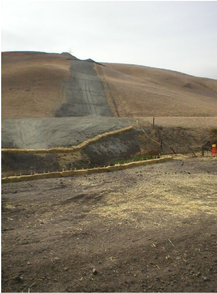
Figure 2 – Long slope over Cayetano Creek lacks adequate BMPs to address erosion prevention and sediment control – November 2 nd .
