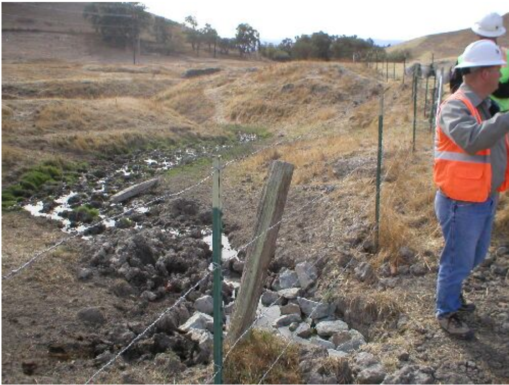
Figure 7 – French Drain installation resulting in diverted flow down a drainage channel from a nearby wetland area - November 2 nd .
