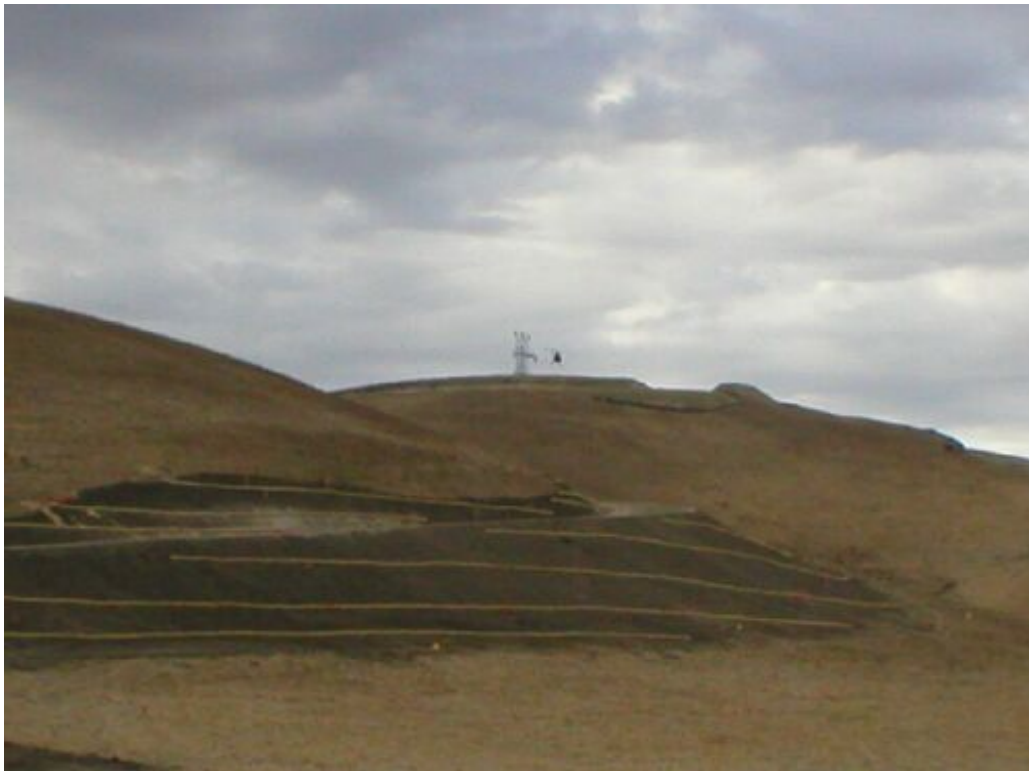
Figure 5 – Rope and line pulling at Tower 13. Note the helicopter to the right of the tower, November 10 th .
