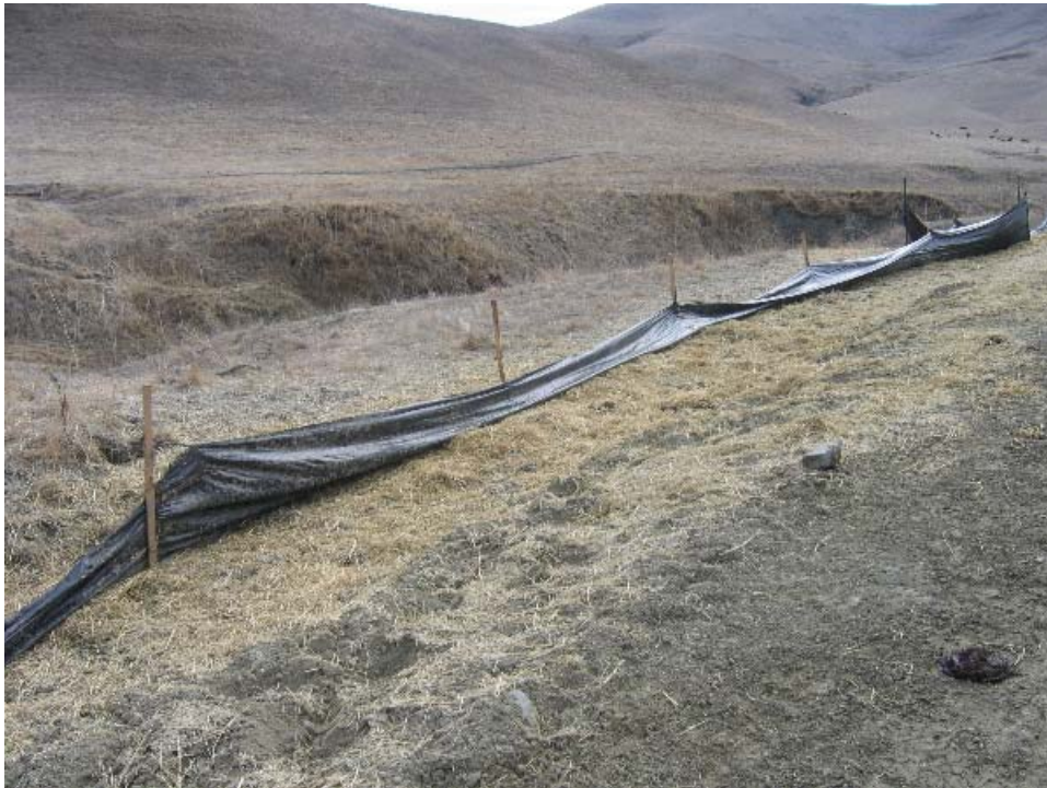
Figure 2 – Sediment fencing in need of repair along the MSA Road, November 28, 2005.
