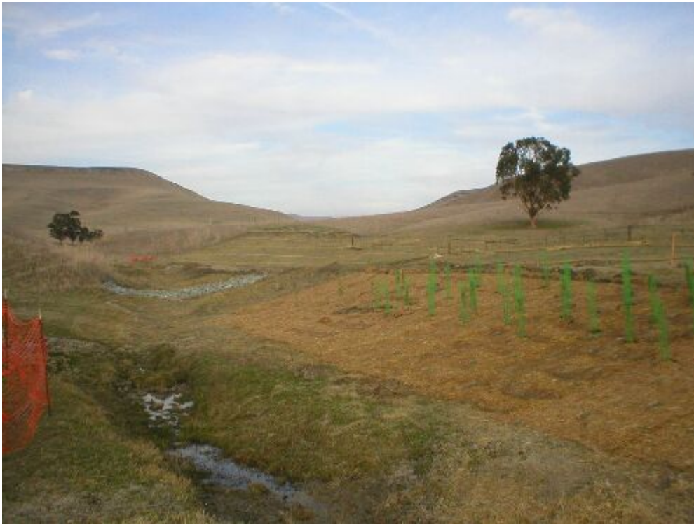
Figure 3 – Monofilament matting installation adjacent to the drainage within the mitigation site, December 14, 2005.
