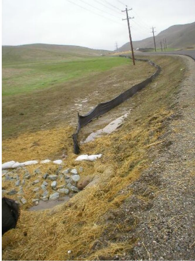
Figure 3 – V-ditch erosion near a culvert along Moller Road, December 29, 2005.
