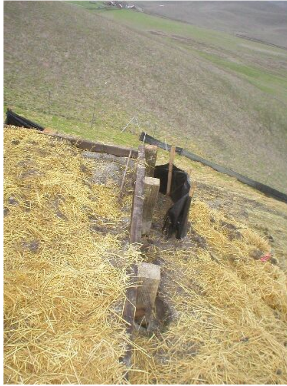
Figure 1 – Erosion at the transition station bulkhead, December 29, 2005.
