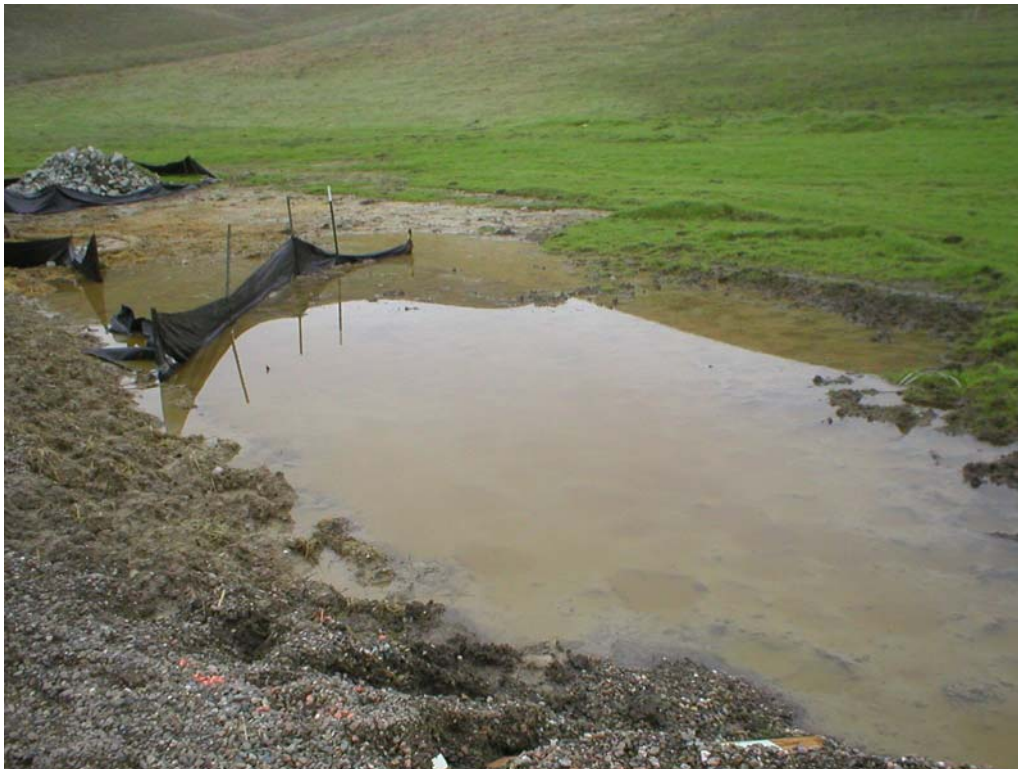
Figure 2 – Ponded area located along Moller Road, near the substation, December 29, 2005.
