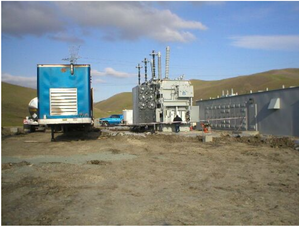
Figure 7 – Transformer being prepared for mineral oil fill at the North Dublin Substation, January 25, 2006.
