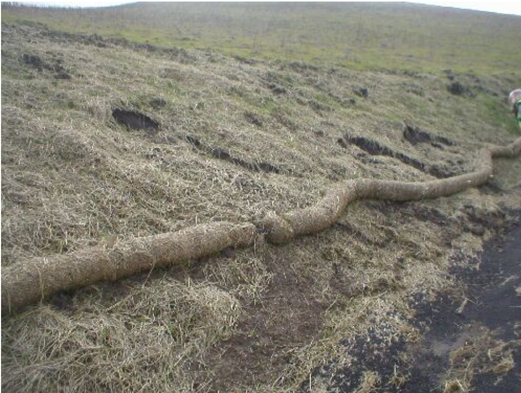
Figure 2 – Slumping along the graded area above Road 6, January 27, 2006.
