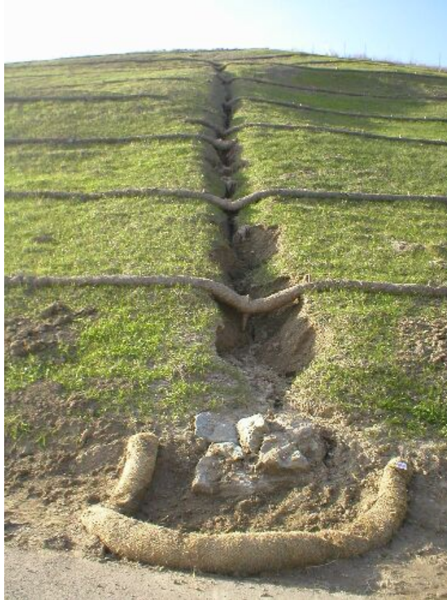
Figure 5 – Continued erosion issue along Moller Road, January 25, 2006.
