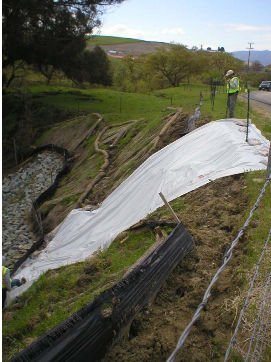
Figure 1 – NVC crews installed fencing and visquene along the Tassajara Creek bank stabilization area, April 7, 2006.
