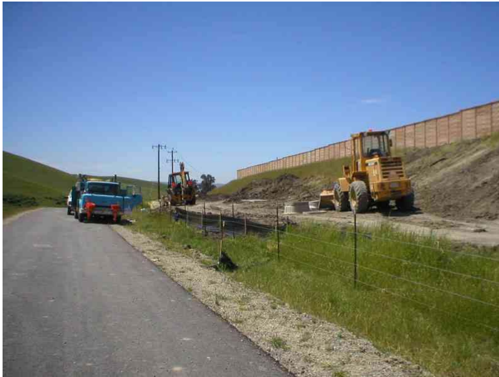
Figure 5 – “Gas-stubbing” and communication vault work adjacent to the North Dublin Substation, May 15, 2006
