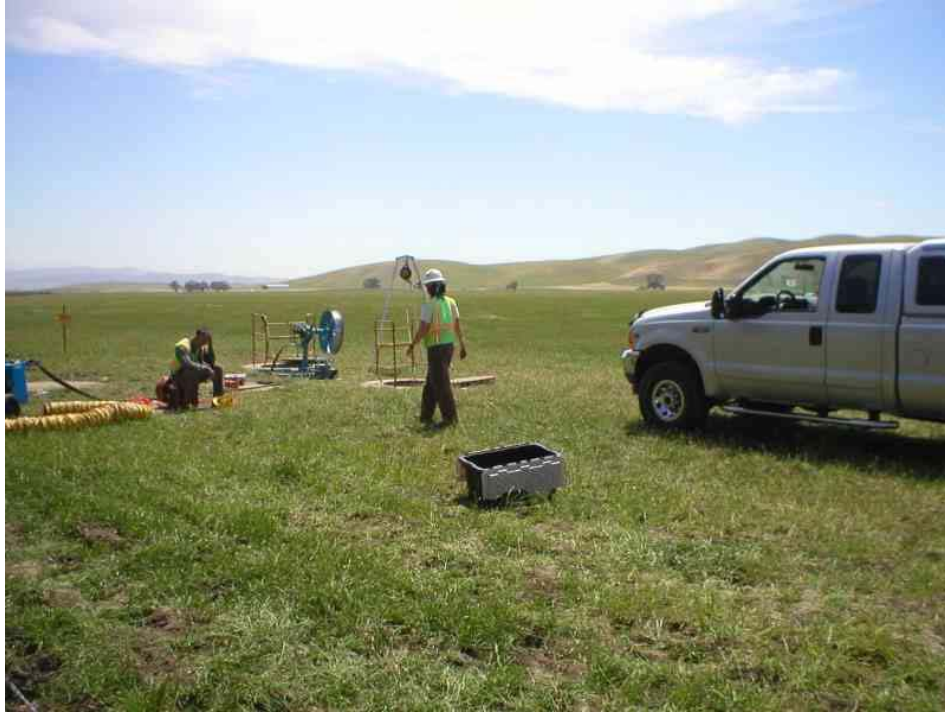
Figure 1 – Ranger crews proofing the conduit by pulling a mandrill at the Vault 2 location, May 15, 2006.
