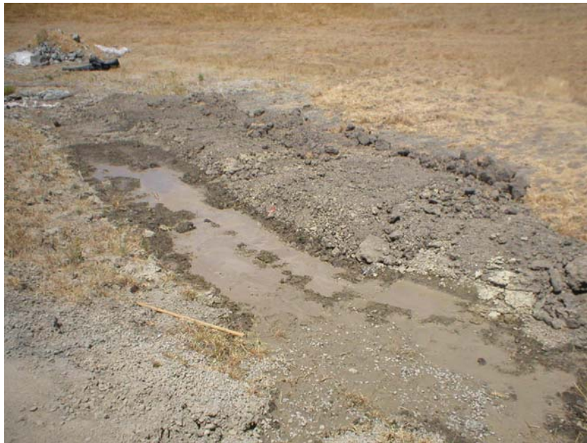
Figure 5 – Dirt placed in a depression which had shown significant ponding along Moller Road. June 30, 2006.
