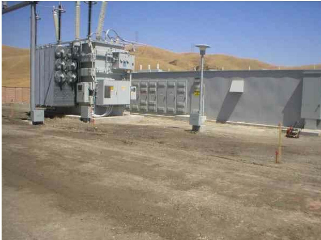
Figure 3 – Transformer at the North Dublin Substation, August 3, 2006. Note that the secondary containment berm around the transformer has been dismantled.
