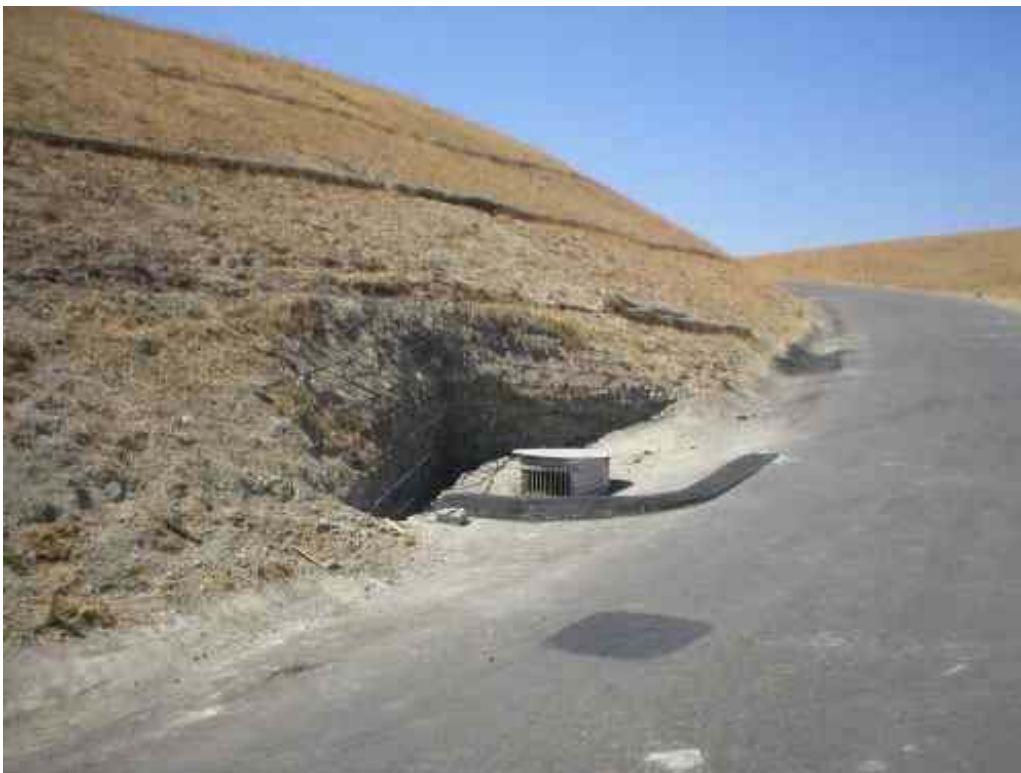
Figure 6 – NVC Crews set a steel cage at a culver inlet along Road 6, September 7, 2006.
