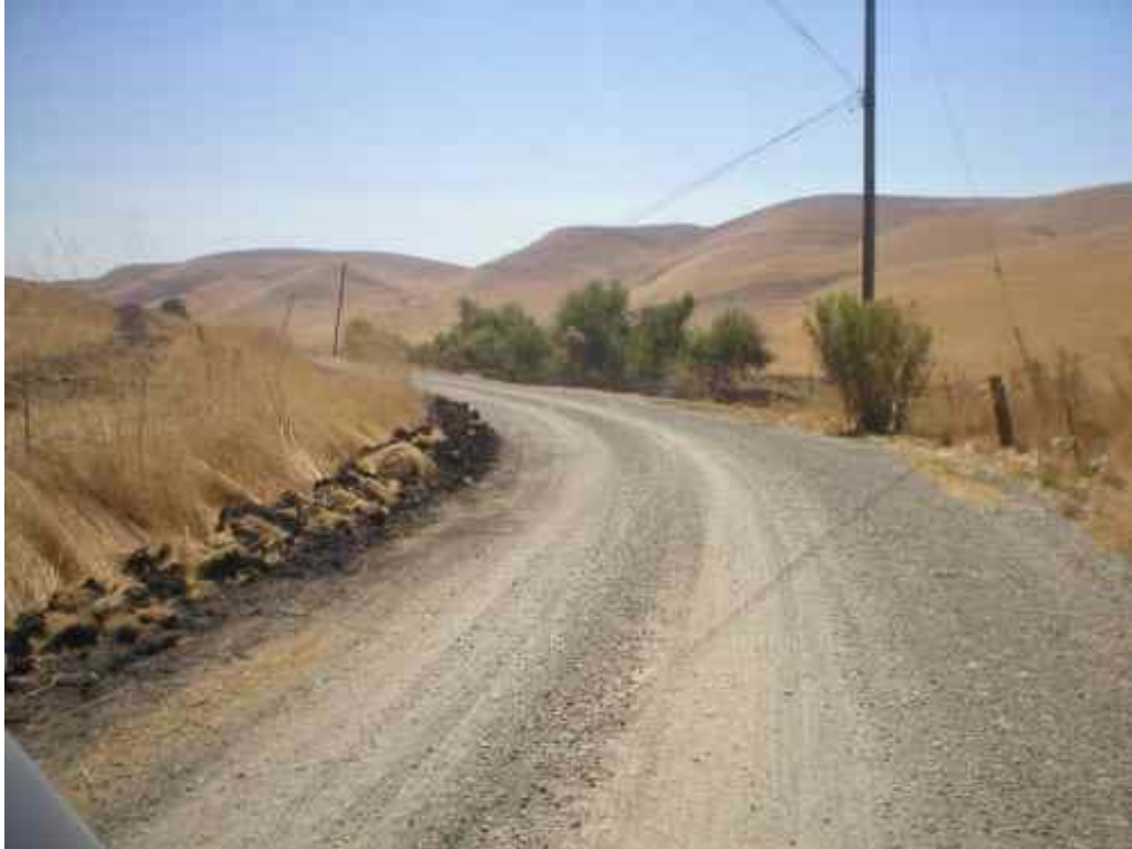
Figure 3 – Loose dirt along Road 5, September 7, 2006.
