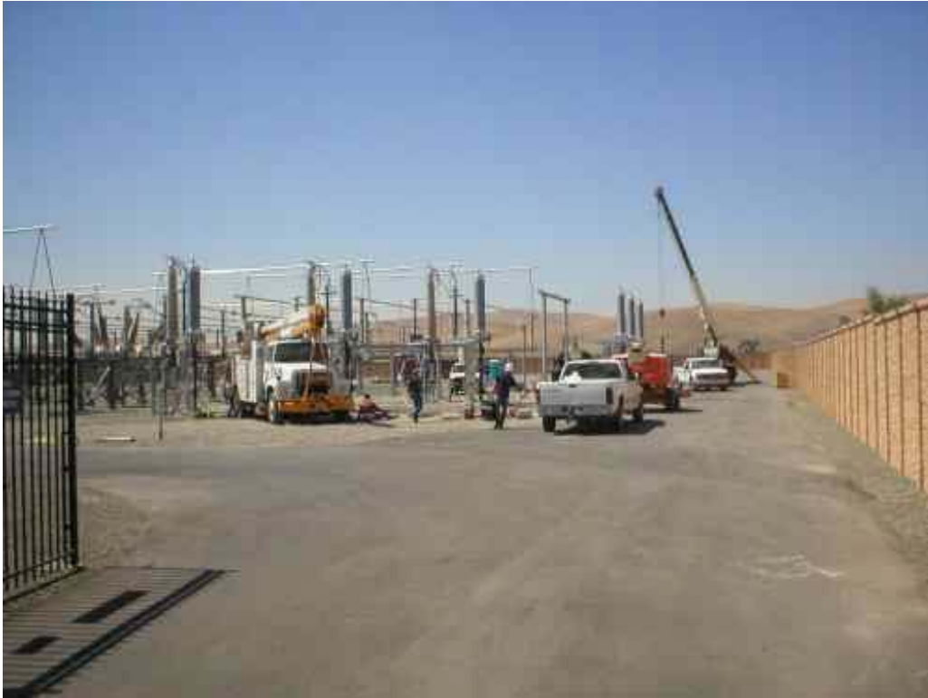
Figure 1 – Nexans crews worked on pothead installation and Wilson crews attached jumpers at the Cayetano Substation, September 7, 2006.
