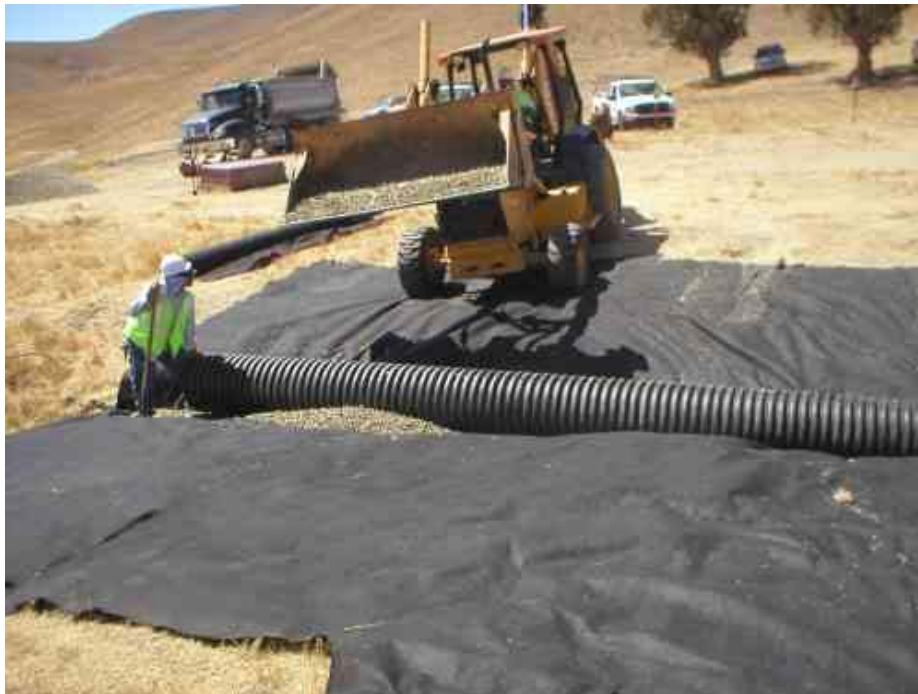
Figure 3 – Temporary culvert installation within the jurisdictional waterway, August 27, 2007. Note the gravel placement over the culvert.
