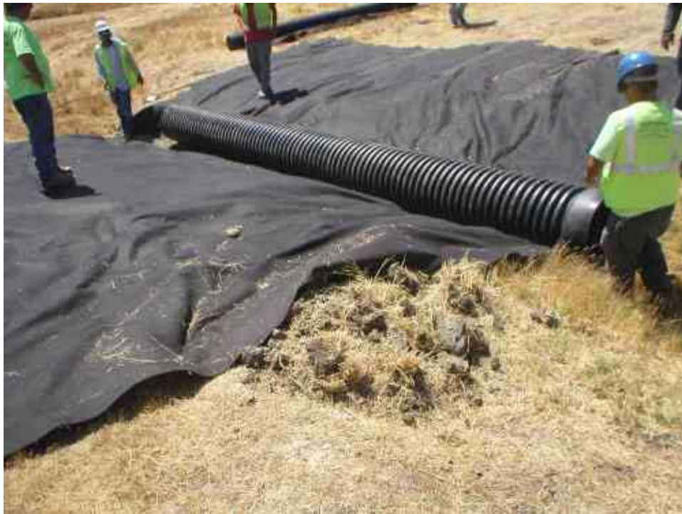
Figure 2 – Temporary culvert installation within the jurisdictional waterway, August 27, 2007. Filter fabric was installed to allow a clean removal post construction.
