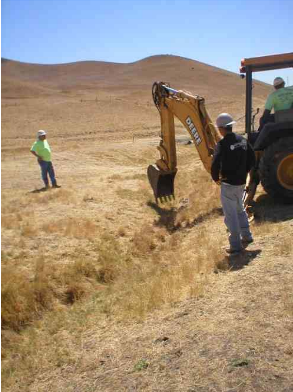
Figure 1 – Temporary culvert installation within the jurisdictional waterway, August 27, 2007. Note that crews are smoothing the drainage bottom to allow a good fit for the culvert.
