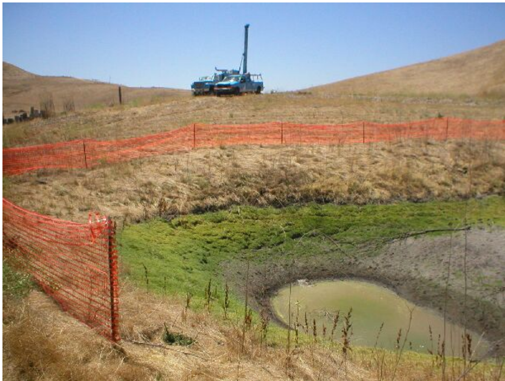
Figure 2 – CTS breeding pond. Note the construction occurring within 200 feet of the resource. Phase Three, July 26, 2005.
