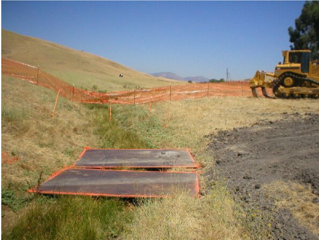
Figure 1 – Bridged drainage off Manning Road. Note the grading near/possibly within the resource. Phase Three, July 26, 2005.
