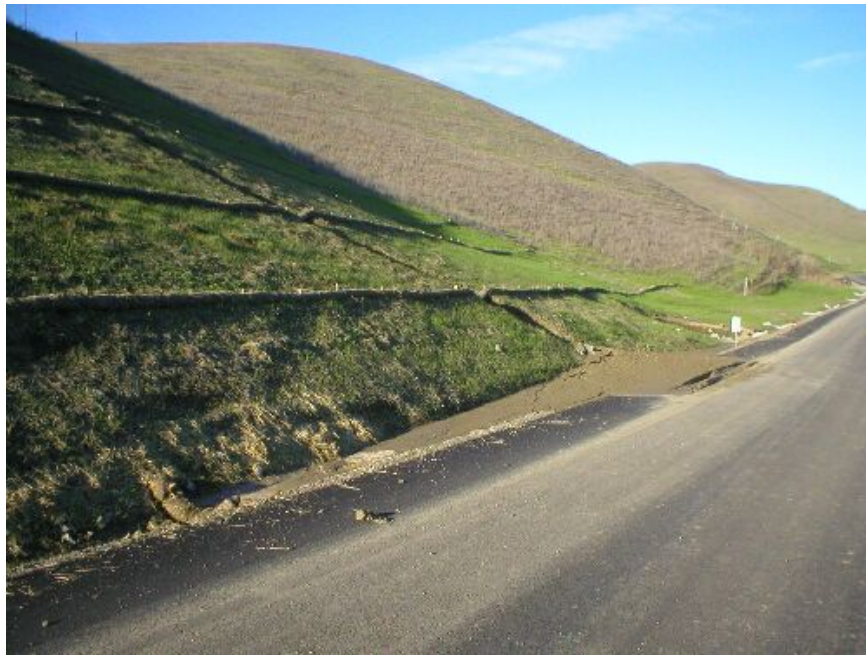
Figure 3 – Erosion from the earthen v-ditch along Moller Road, January 4, 2006.
