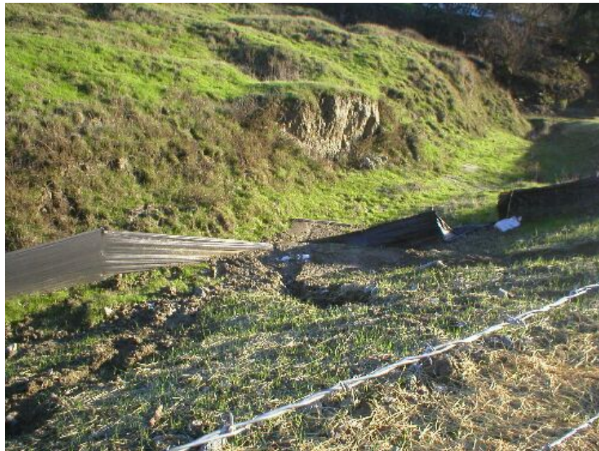
Figure 4 – Overrun sediment fencing along Moller Road upstream of Tassajara Creek, January 4, 2006.
