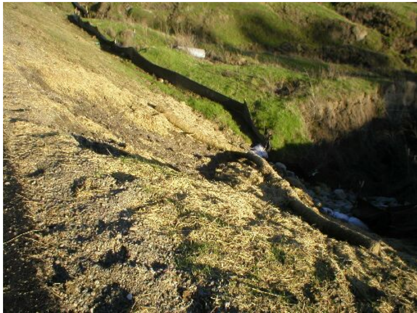
Figure 5 – Small landslide at a culvert outlet along Moller Road, January 4, 2006.
