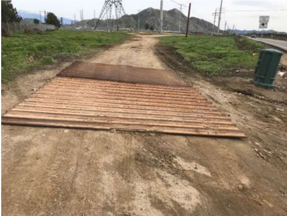
Photo 1 – Shaker plate for track-out control was delivered to the Valley Substation Yard driveway.
