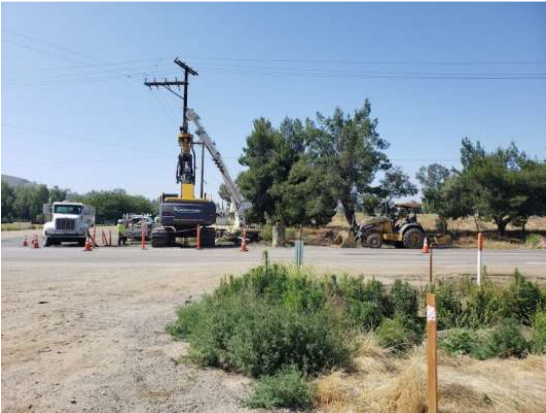
Photo 3 – Traffic control established along Scott Road during drilling at Construction Area UNK155 (June 5, 2019).
