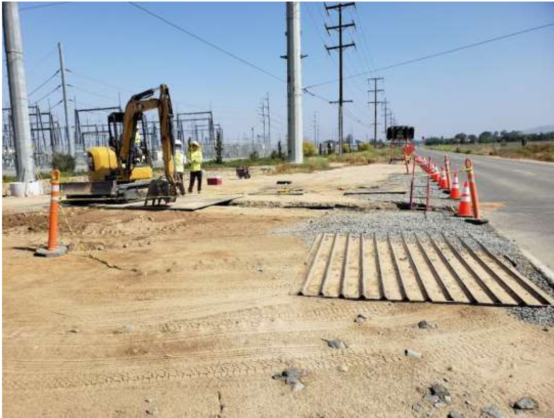
Photo 5. Un-stabilized construction entrance on west side of Menifee Road near the underground trenching (June 18, 2019).
