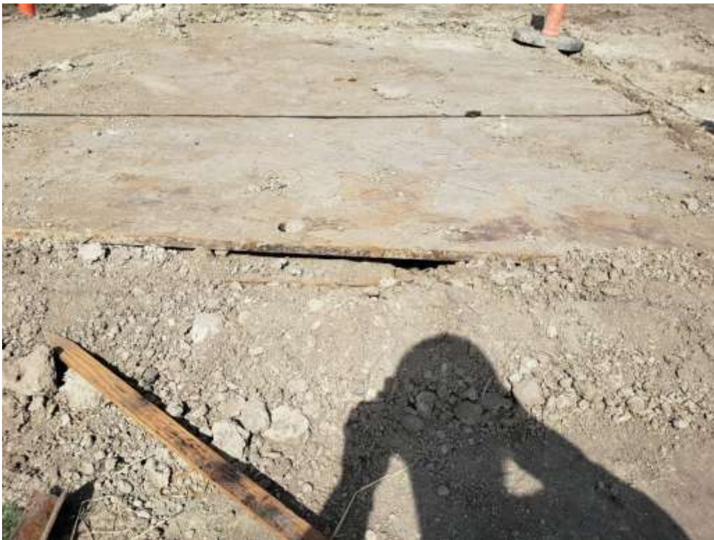
Photo 4 – Gaps between covering and excavation hole at Construction Area UNK155 (June 18, 2019).
