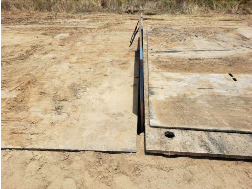
Photo 3 – Vault #3 excavation with gaps in steel plate coverings (June 11, 2019).
