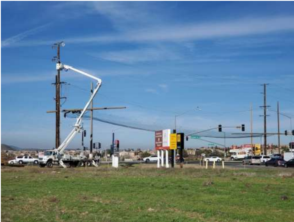
Photo 3 – Wire stringing activities at Construction Area UNK235 showing netting over Winchester Road (January 15, 2020).
