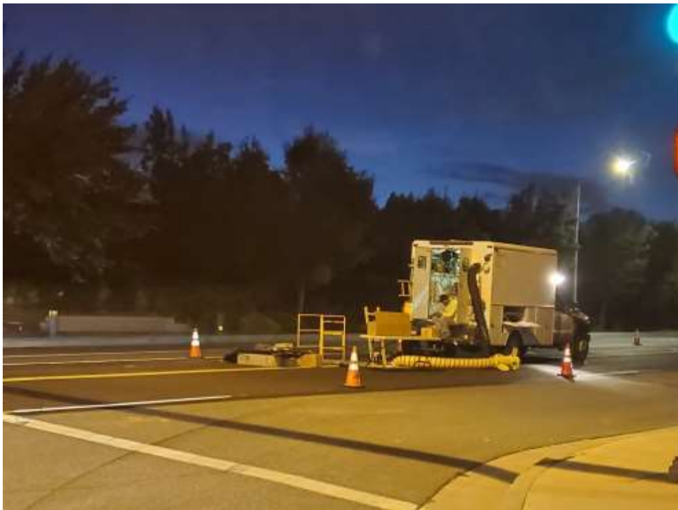
Photo 2 – SCE self-perform crews conducting overnight underground work on Leon Road between Construction Areas UNK207 and UNK222 (July 21, 2020).
