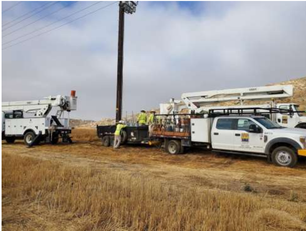
Photo 1 – Wilson crews preparing to install capacitor bank at Construction Area UNK66 (July 14, 2020).
