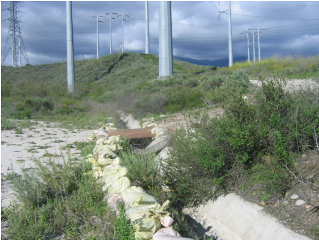
Photo 3: Area behind the Viejo Substation where a v-ditch was installed for drainage.
