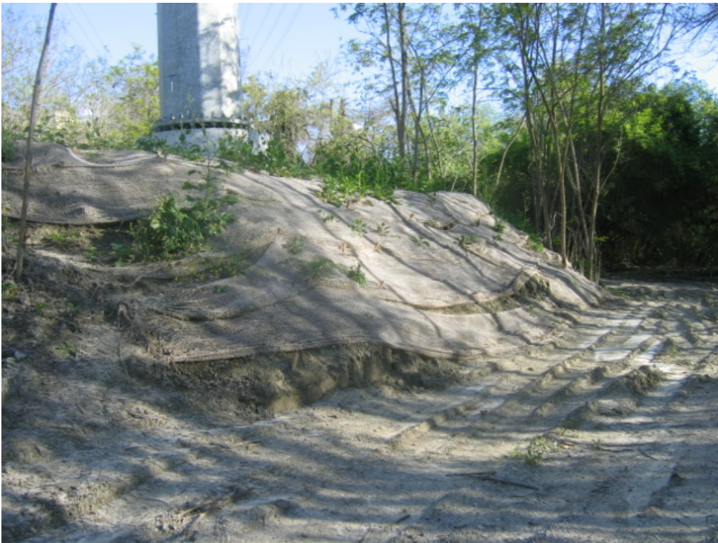
Photo 5: Restored area near Chiquita Substation. Jute netting was used to stabilize the slope leading to the tower pad.
