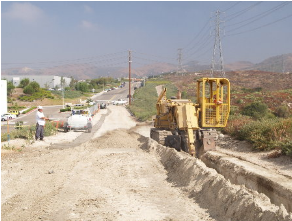
Figure 4 – Trenching machine operating down access road for future 66 kV connection. Utility connection already made and trench backfilled with a grout slurry (see trenchline along the roadway).
