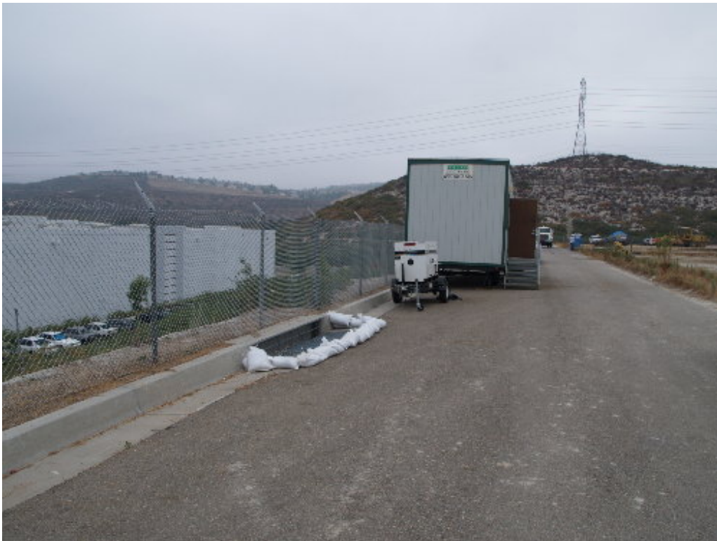
Figure 3 – Sandbags placed around storm drains. Filter fabric will be placed over drain and secured by the sandbags.
