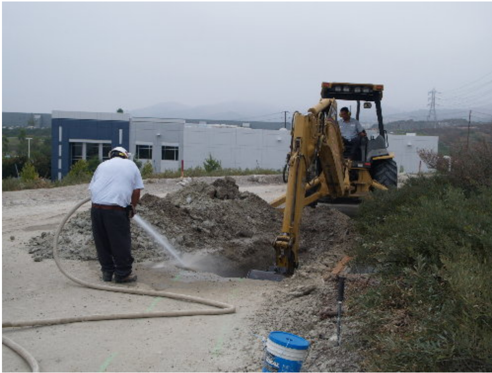
Figure 5 – A trailer-mounted water system was used to control fugitive dust during the trenching operation.
