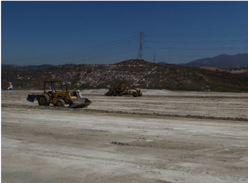
Figure 3 – Operators worked with a motor grader and backhoe to grade the site and remove larger rocks.
