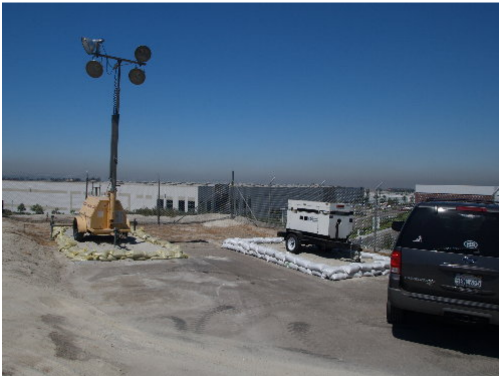
Figure 2 – Containment berm for the portable light plant increased with additional layer of sandbags.
