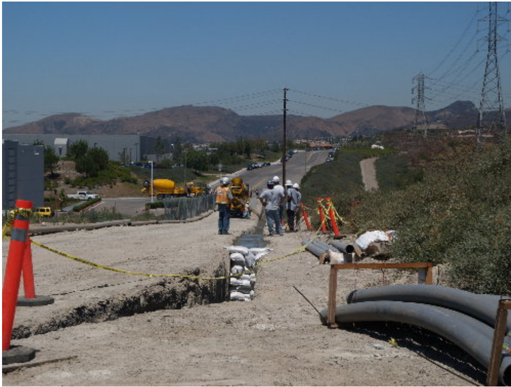
Figure 5 – The electric conduit trench along the access road was being backfilled with concrete slurry.
