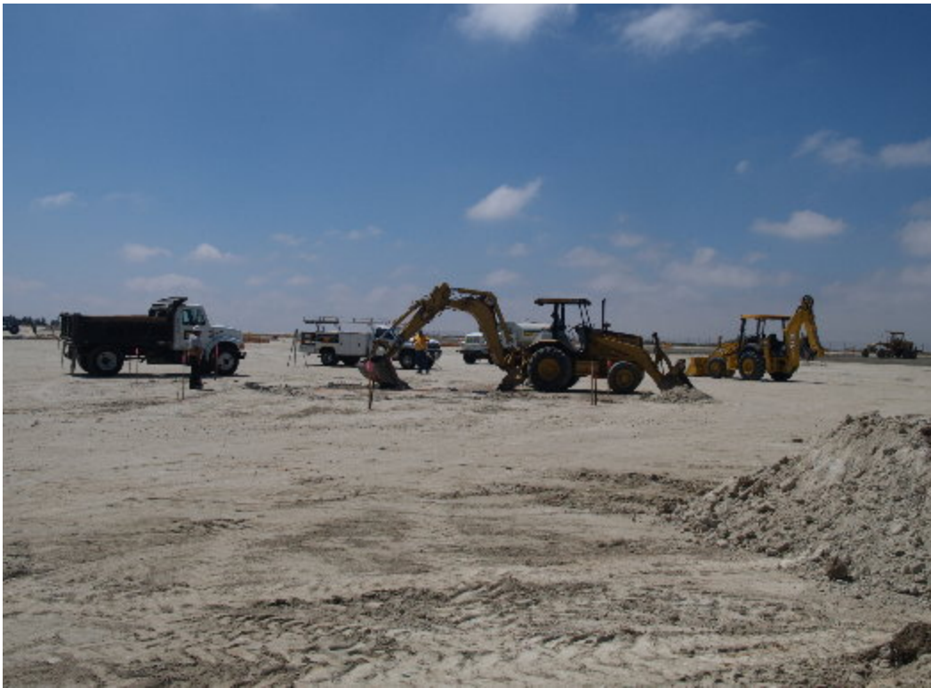
Figure 2 – An operator in a backhoe worked on excavating a foundation site on the north end of the station.
