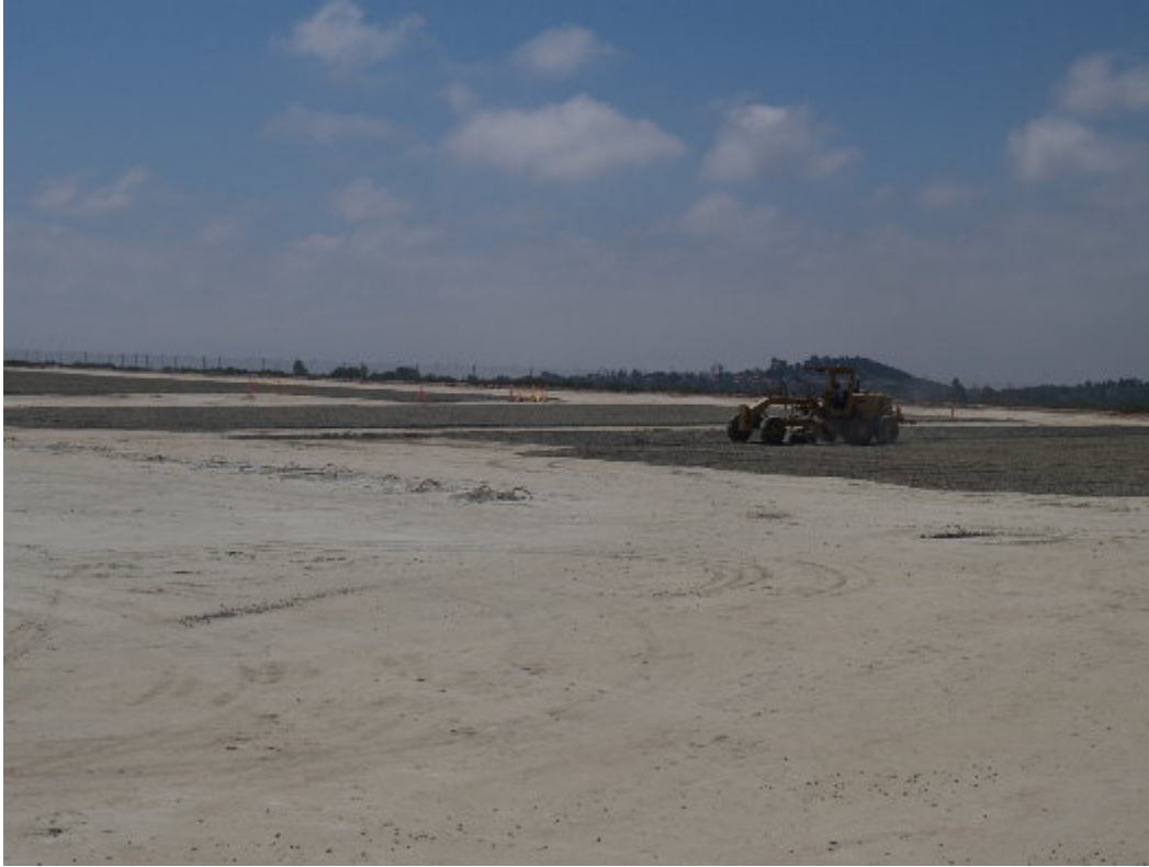
Figure 1 – Rock has been placed over the grounding grid on the substation site and is being spread by an operator in a motor grader.
