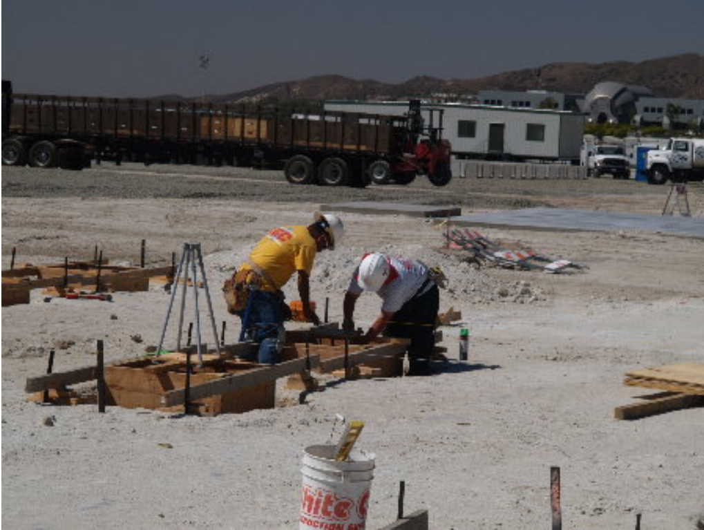
Figure 1 – Crews working on the form work and anchor bolts for the foundation pilings at the substation site.
