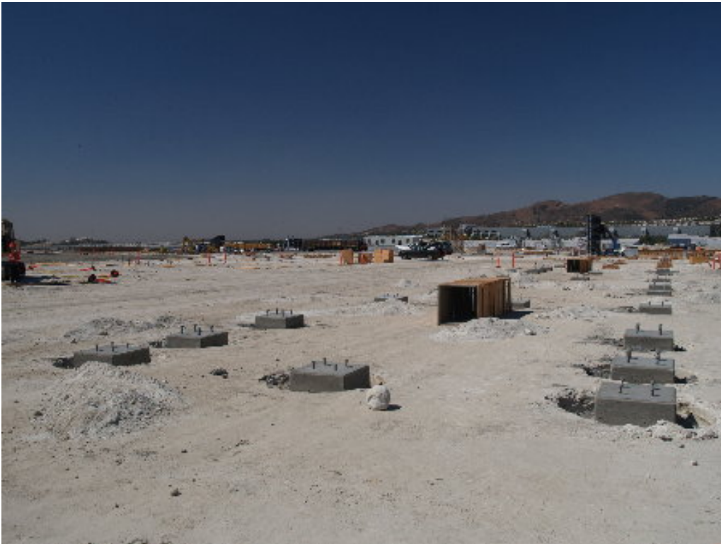
Figure 2 – Completed foundation pilings with anchor bolts. Most structures at the substation site will rest on raised foundations.
