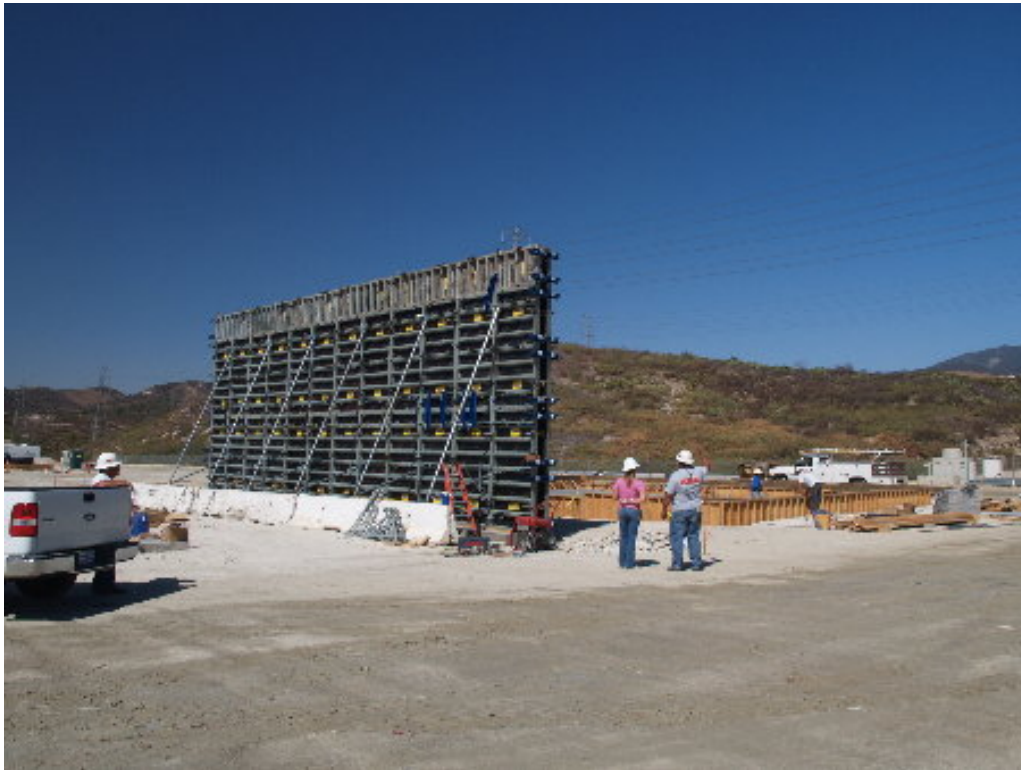
Figure 3 – The reusable form for the vertical firewall that will separate one of the two A transformers (230 kV) and the electrical building has been set up and is ready for the concrete pour.
