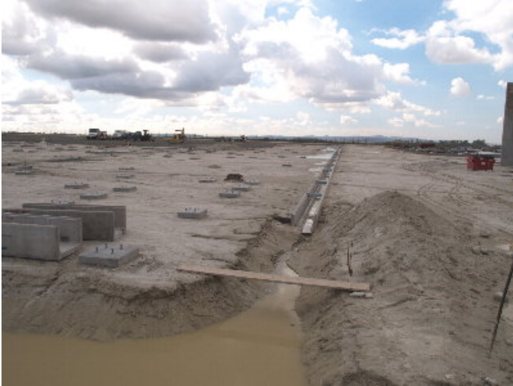
Figure 1 – The pre-formed concrete trenches were set during the week despite the rain. Note the final two pre-form pieces sitting above the trench to the left.
