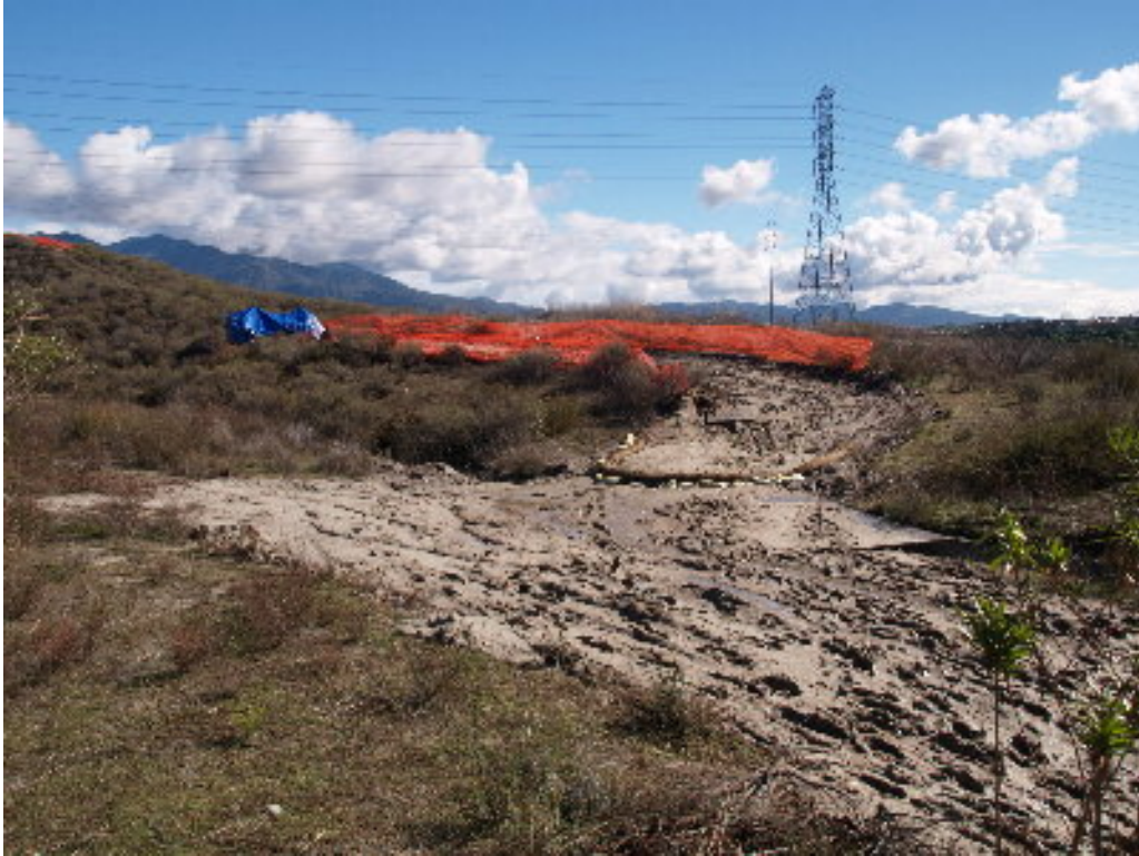
Figure 3 – Sediment flowing down from a pad on the transmission line right-of-way toward the concrete drainage ditch.
