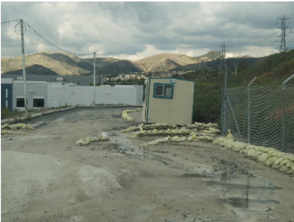
Figure 2 – Additional rows of sandbags were placed near the guard shack to control the large amount of water run-off and sediment. The rear of the guard shack settled in the saturated soil.
