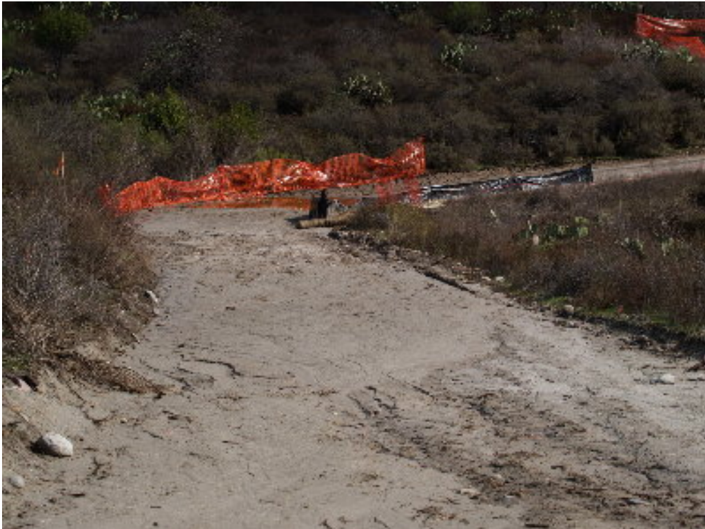
Figure 4 – Water from the natural drainage and from along the access road has settled in the low area at the crossing.
