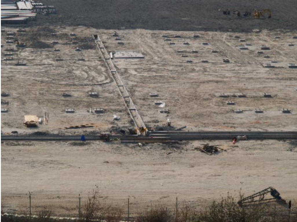
Figure 1 – Crews continued working on the preparation of the pre-cast concrete electrical trenches on the substation site.
