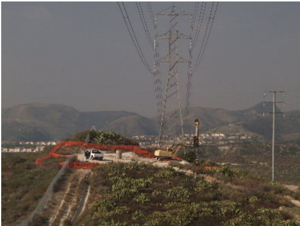
Figure 4 – The drilling crew worked on the last foundations for the tower east of the substation site on the 220 kV transmission line corridor.
