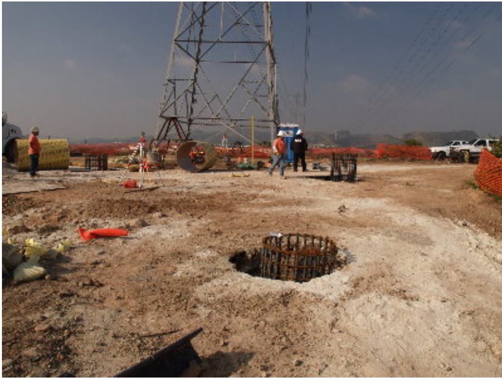
Figure 5 – A crew set rebar cages in the lattice tower foundation excavations on the hill southeast of the substation site.
