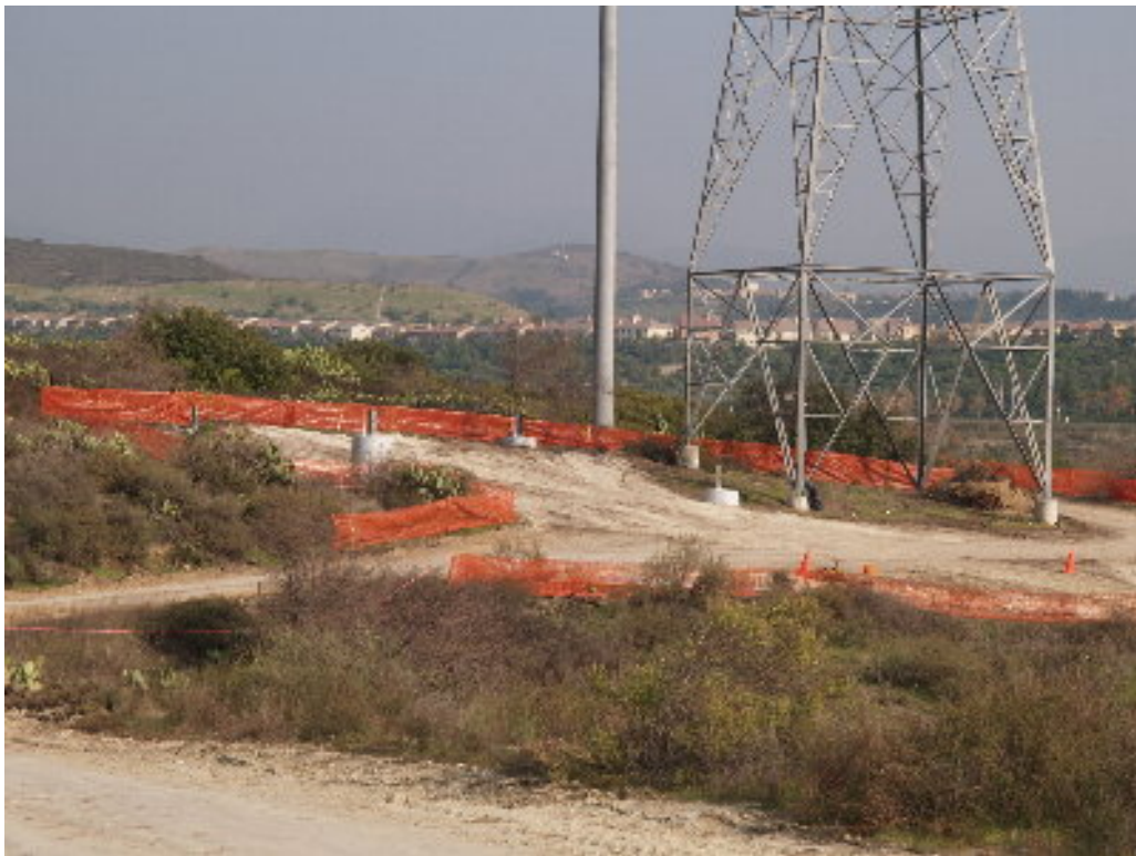
Figure 6 – The foundation for the lattice tower at the base of the hill southeast of the substation site has been completed. Note the size compared to the existing lattice tower.
