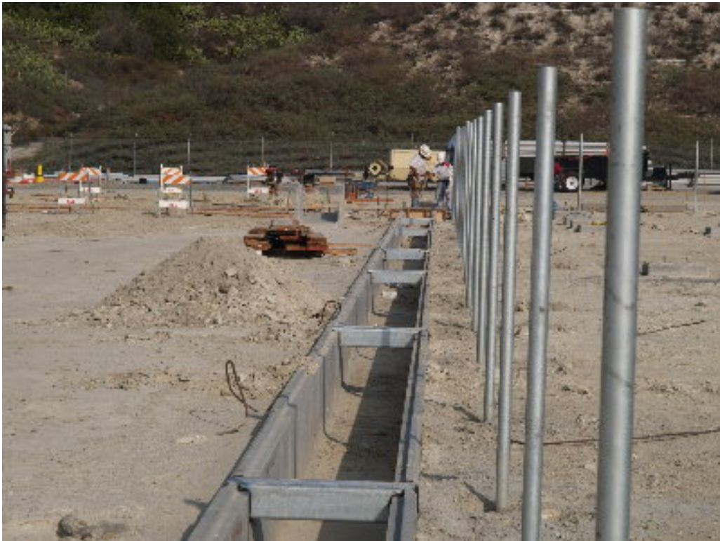
Figure 2 – Metal braces for the grate system were set on some of the pre-cast concrete electrical trenches on the substation site.
