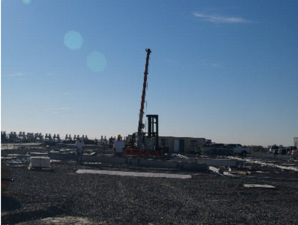
Figure 1 – A small crew worked to connect conduits to the pre-cast trench on the southern end of the substation site.
