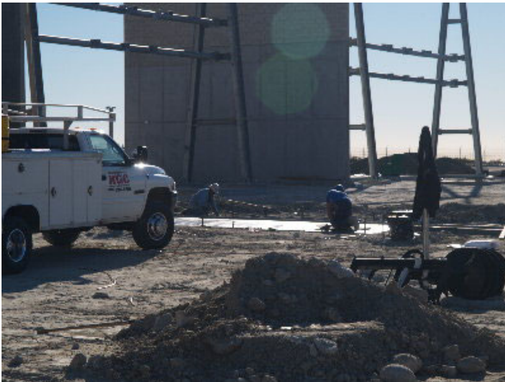
Figure 2 – A crew worked on finishing the concrete slab outside the northern wall of MEER #1.
