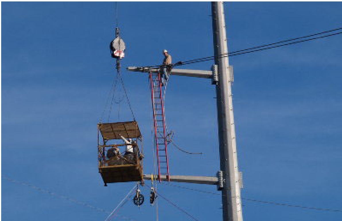
Figure 4 – The Hill Crane held a basket to allow workers to connect cables and insulators to the steel pole arms.
