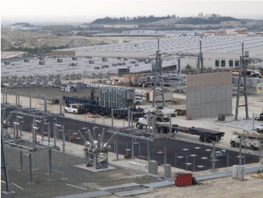
Figure 1 – Crews prepared the pad and the first A transformer for the lift onto the pad.
