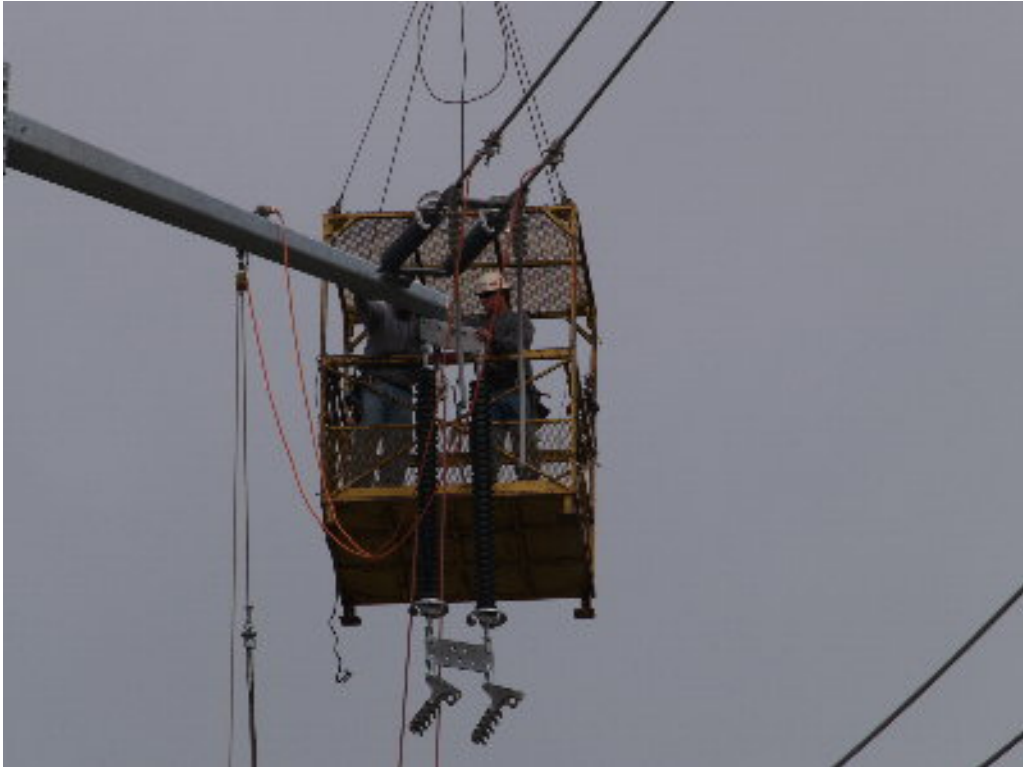
Figure 4 – The Hill Crane held a basket to allow workers to connect cables and insulators to the steel pole arms.
