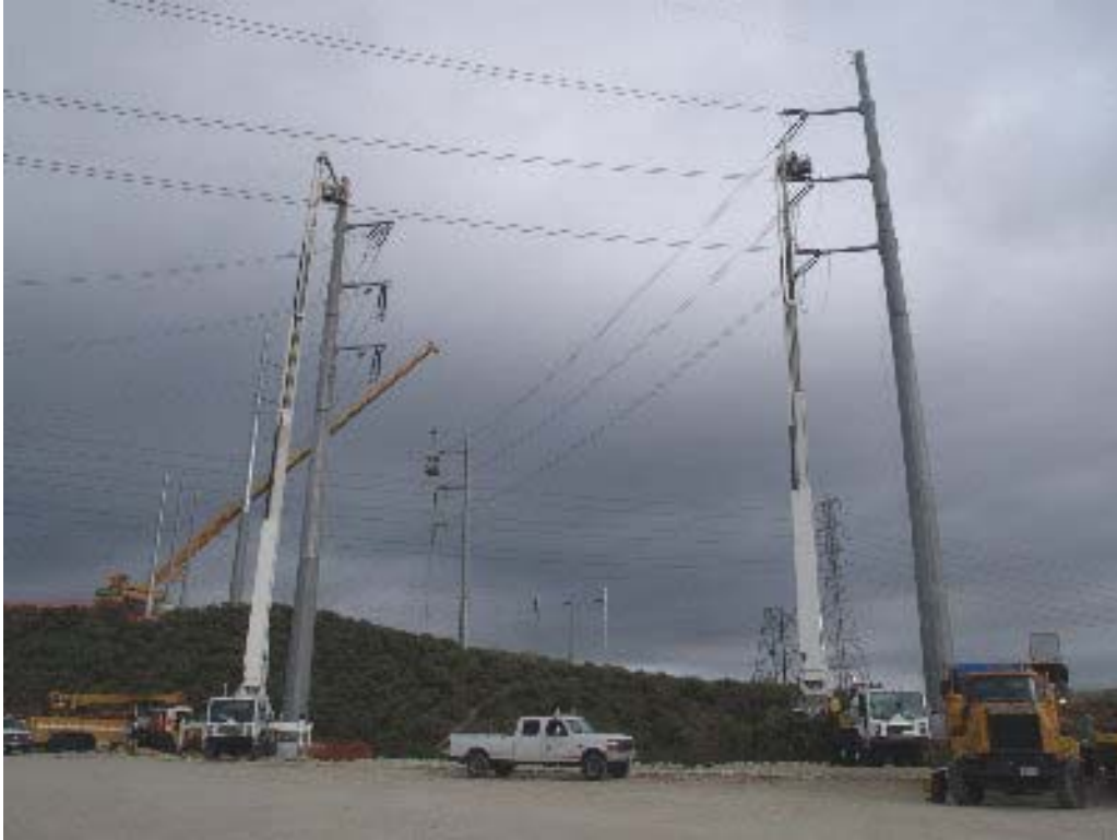
Figure 5 – Two man-lifts were used to string cable between the transmission line corridor and the substation. Cables are now connected to the large A-frame supports within the substation site.
