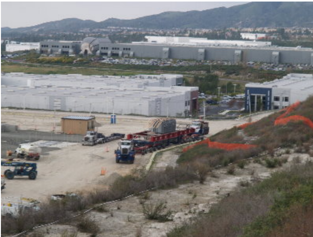
Figure 2 – A special truck was used to move the transformers within the substation site. Note the size difference against the normal tractor-trailer to the left.
