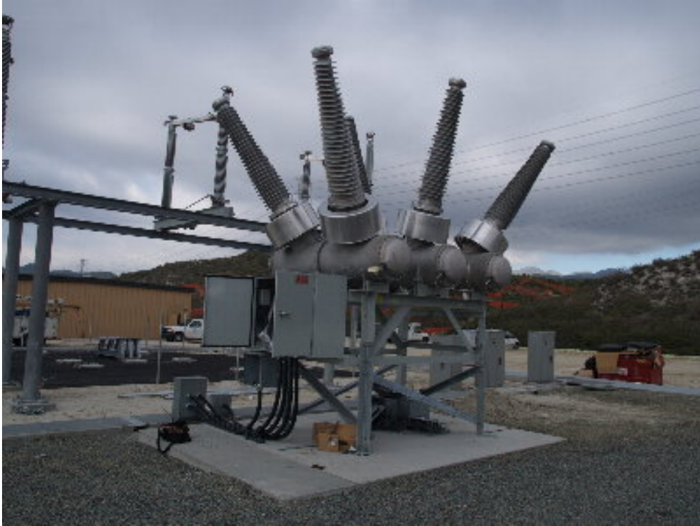
Figure 3 – Most of the equipment has been delivered to the substation site and set on completed foundations.
