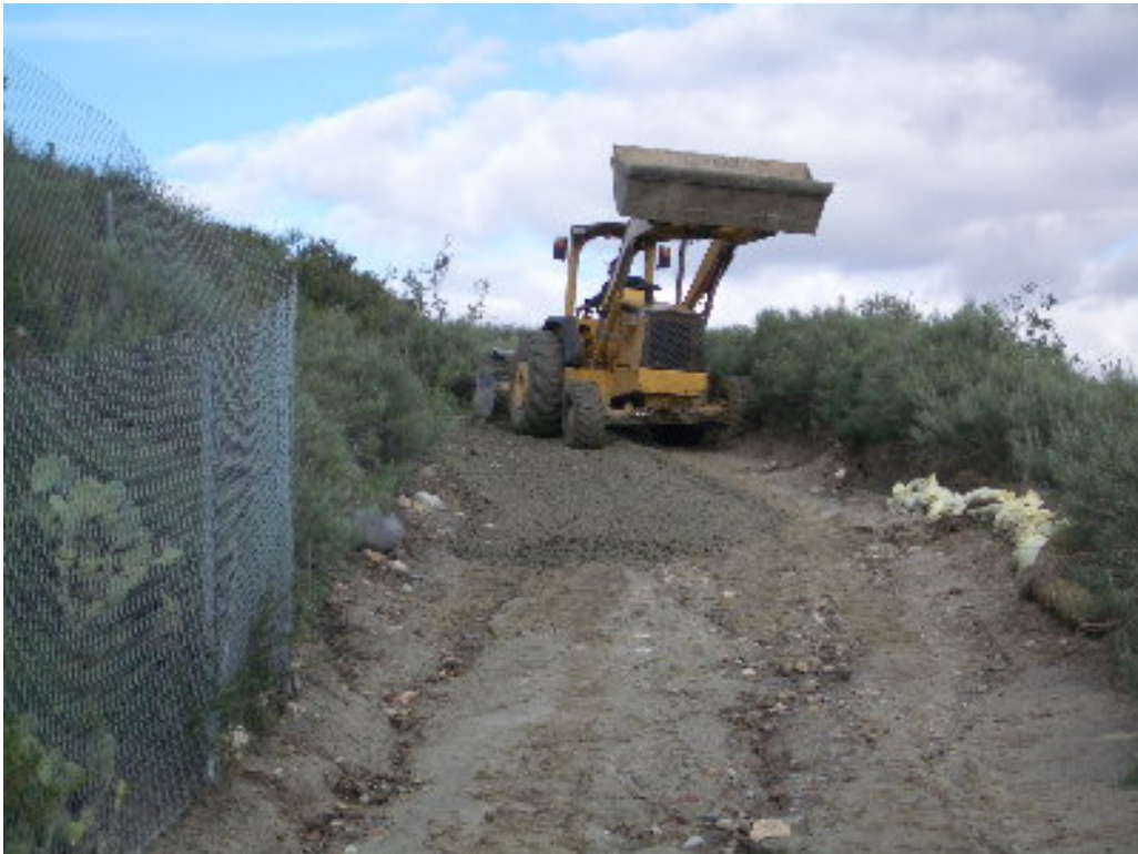
Figure 4 – Rock was spread on the 220 kV access road to address erosion and provide all-weather access.
