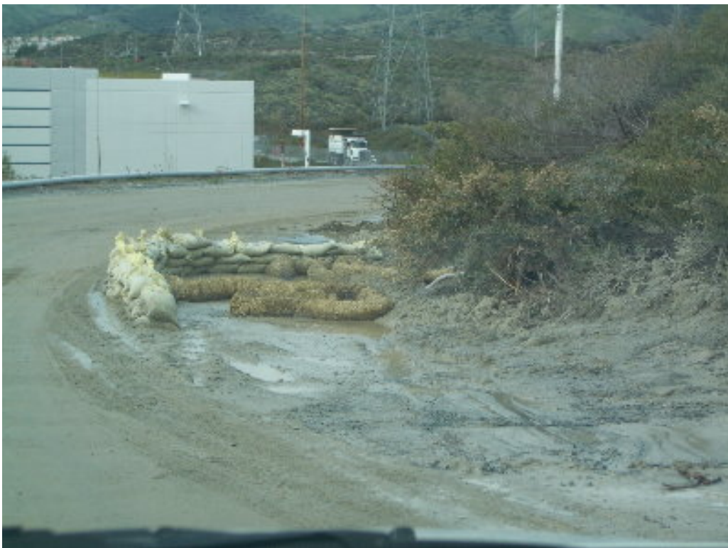
Figure 2 – The BMPs at the storm drain on the access road were repaired.
