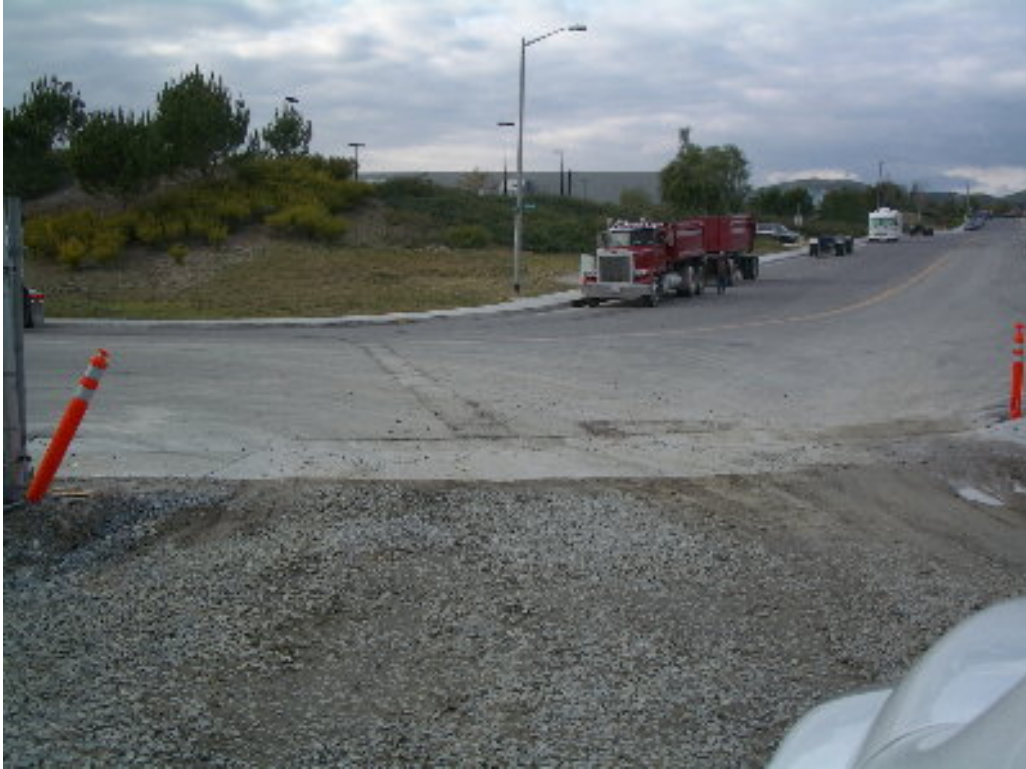
Figure 3 – Material tracked onto the public right-of-way will be cleaned prior to the predicted rains.
