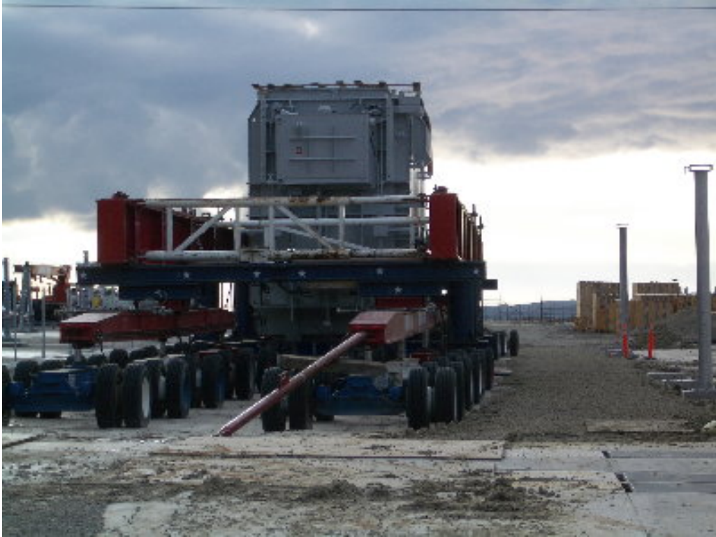
Figure 1 – Crews have spread rock around the truck holding the second A transformer and will set it onto the pad after the predicted rain.
