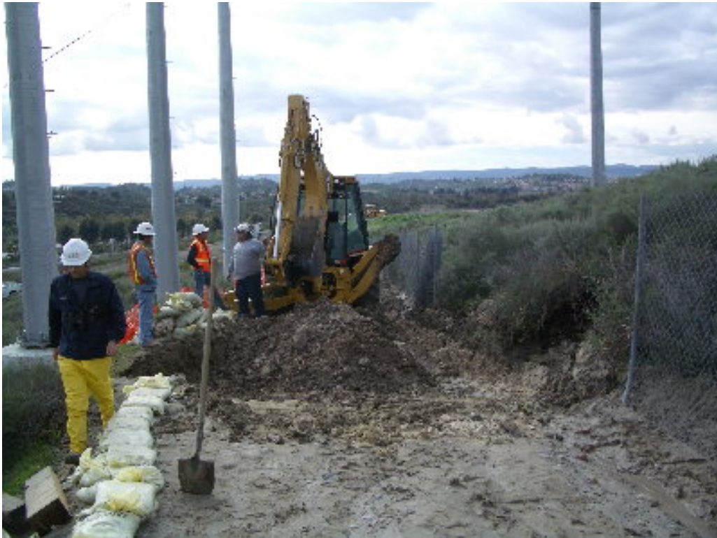
Figure 5 – A crew prepared the pad for the Bronto man-lift under the supervision of the LSA EI.
