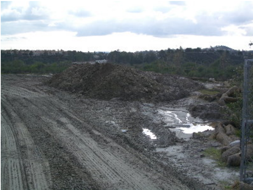
Figure 6 – The spoil pile needs to be addressed and BMPs are required at the culvert crossing near the substation back gate.
