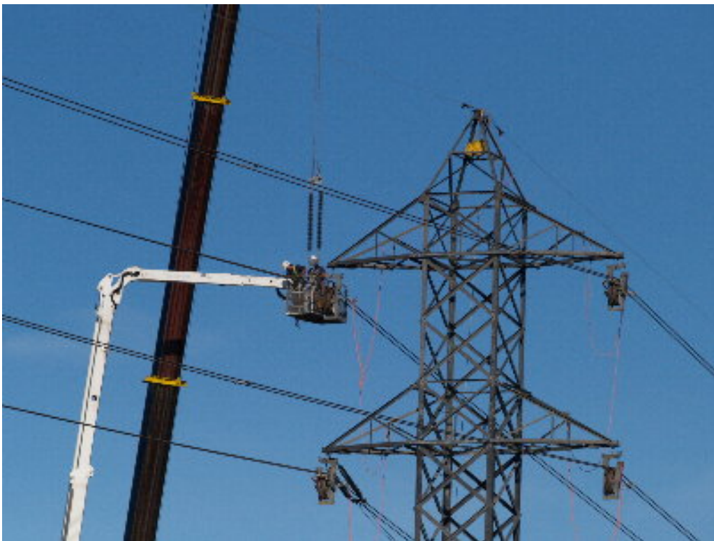
Figure 4 – The transmission line crew worked in a man-lift with the help of the crane to attach insulators to the new lattice towers.
