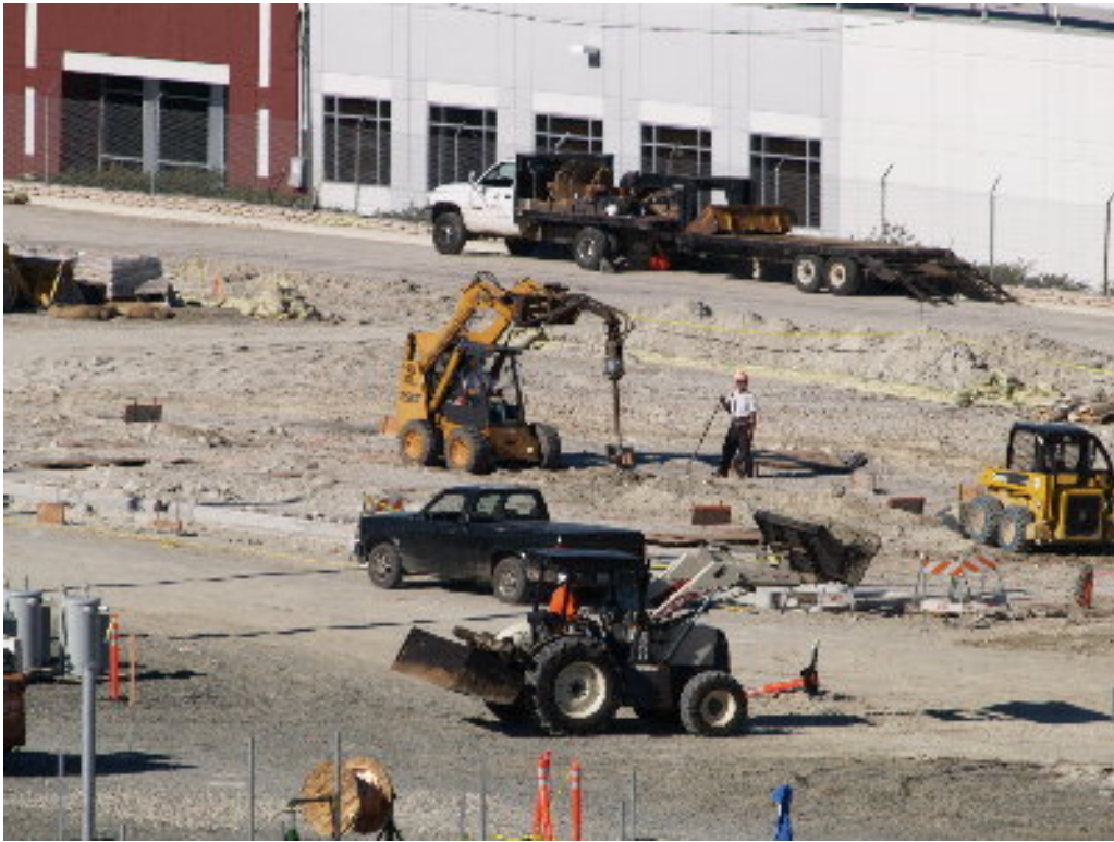
Figure 3 – An operator worked with a Bobcat and small auger attachment to clean out the foundations for the 12 kV structures.
