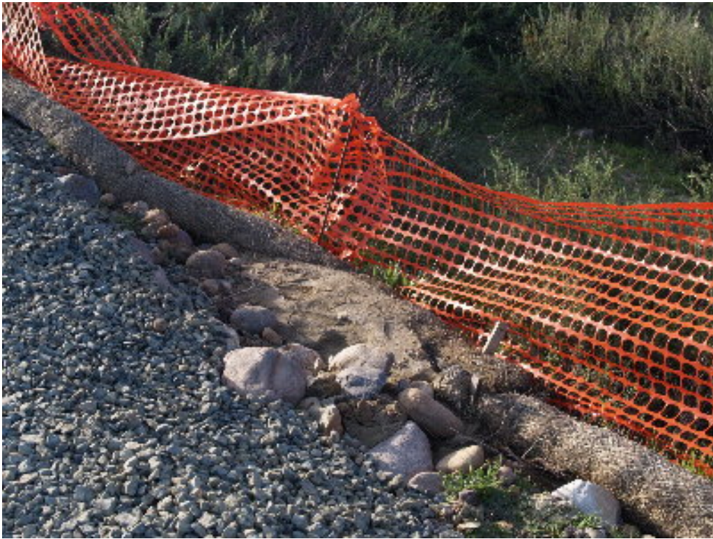
Figure 5 – Several areas on the 220 kV transmission line corridor need BMP maintenance and/or improvement.
