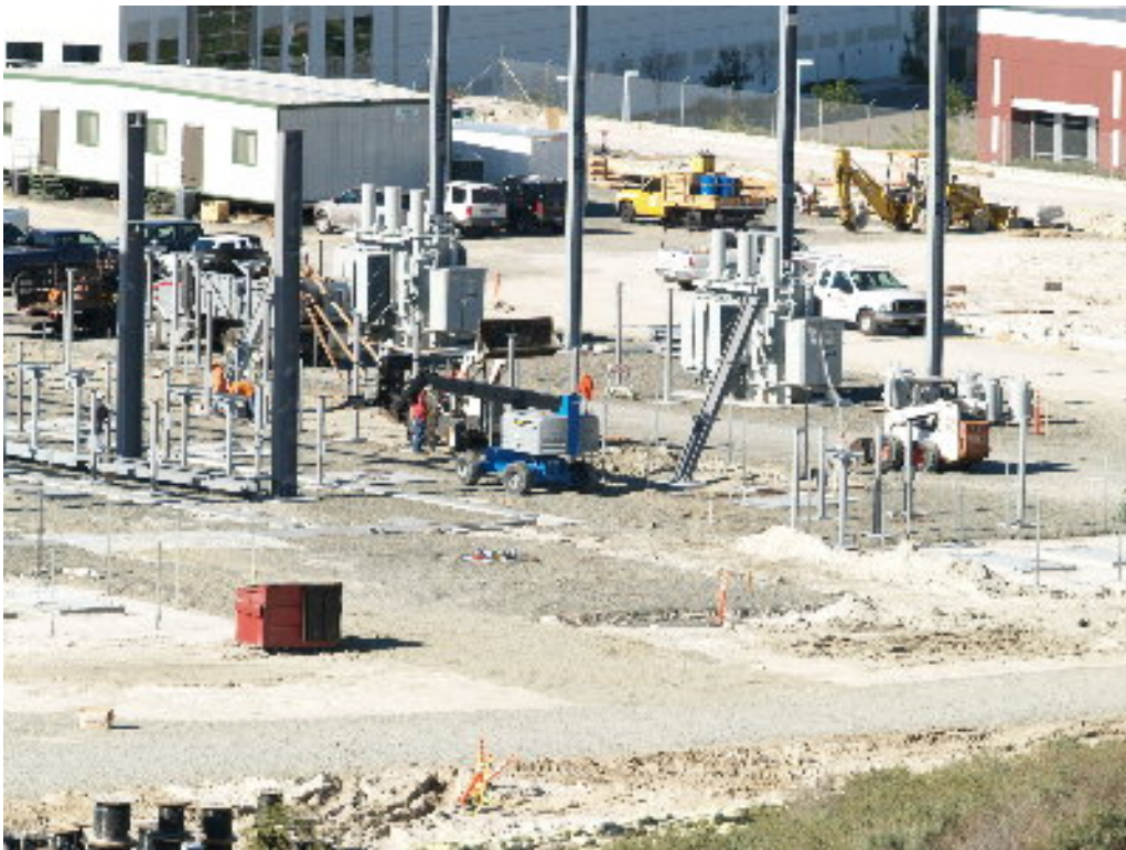
Figure 2 – A crew worked with small lifts to prepare the 66 kV support structures.
