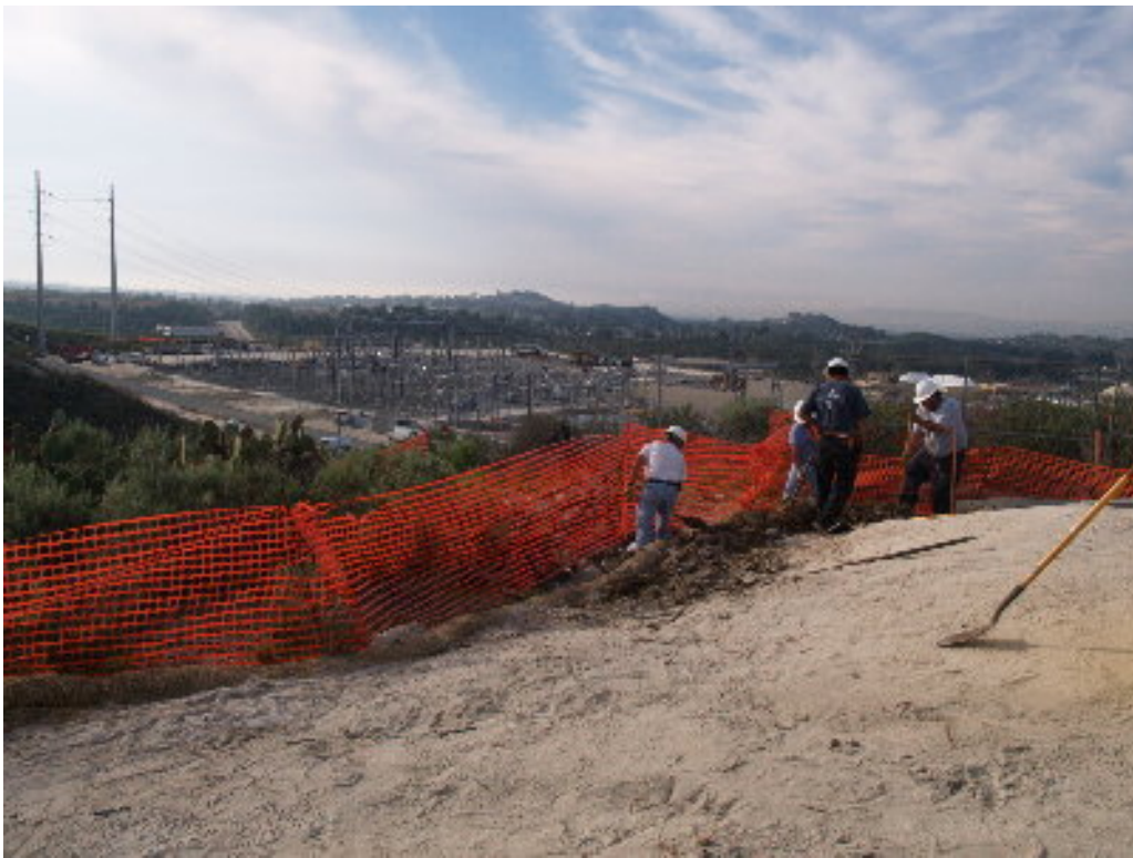
Figure 6 – A small crew installed silt fencing on the 220 kV transmission line corridor.
