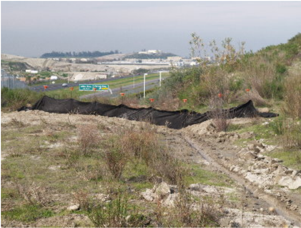
Figure 7 – A dense fabric was used as silt fencing across a small drainage. It will be replaced with appropriate BMPs.
