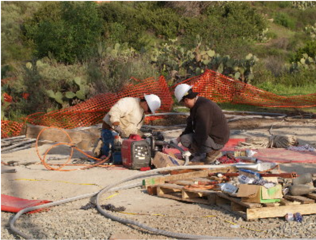
Figure 5 – Workers on the 220 kV transmission line attached connectors to the measured cable.
