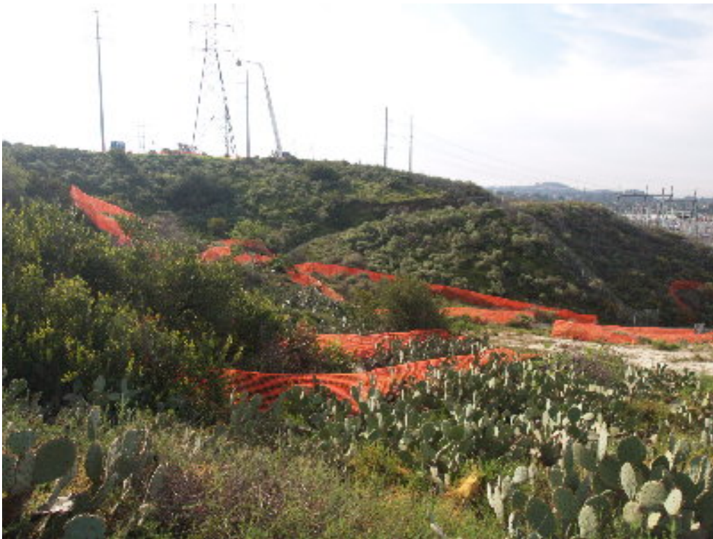
Figure 8 – Biological exclusion fencing has been placed in preparation for construction on the 66 kV segment.
