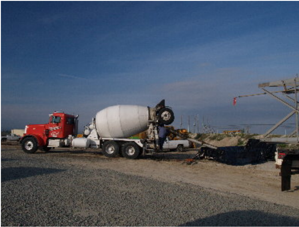
Figure 3 – The concrete drivers correctly washed-out in the prepared area after pouring the 12 kV foundations.
