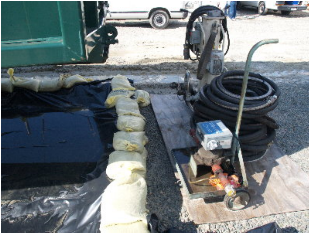
Figure 3 – Containment structures need rainwater or any contaminated water removed and properly disposed.
