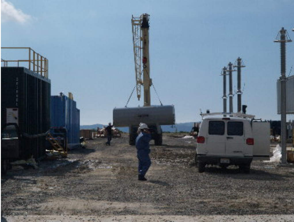
Figure 1 – A SCE crew prepared to install the oil tank on the A-bank transformers.
