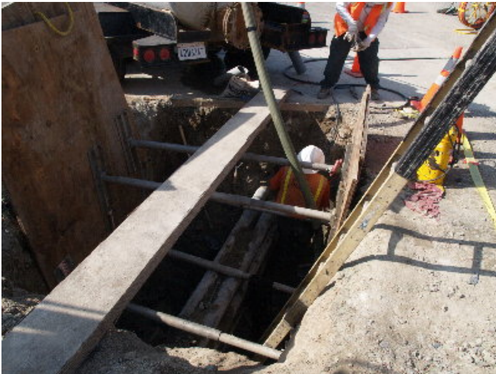
Figure 2 – The PAR crew worked to repair the conduit for the 12 kV power to the substation.
