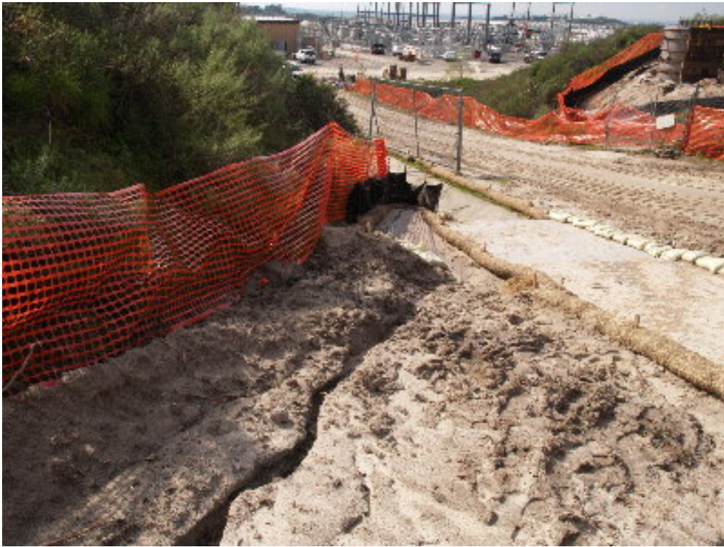
Figure 7 – The BMPs on the 66 kV right-of-way require maintenance before any additional rain events.
