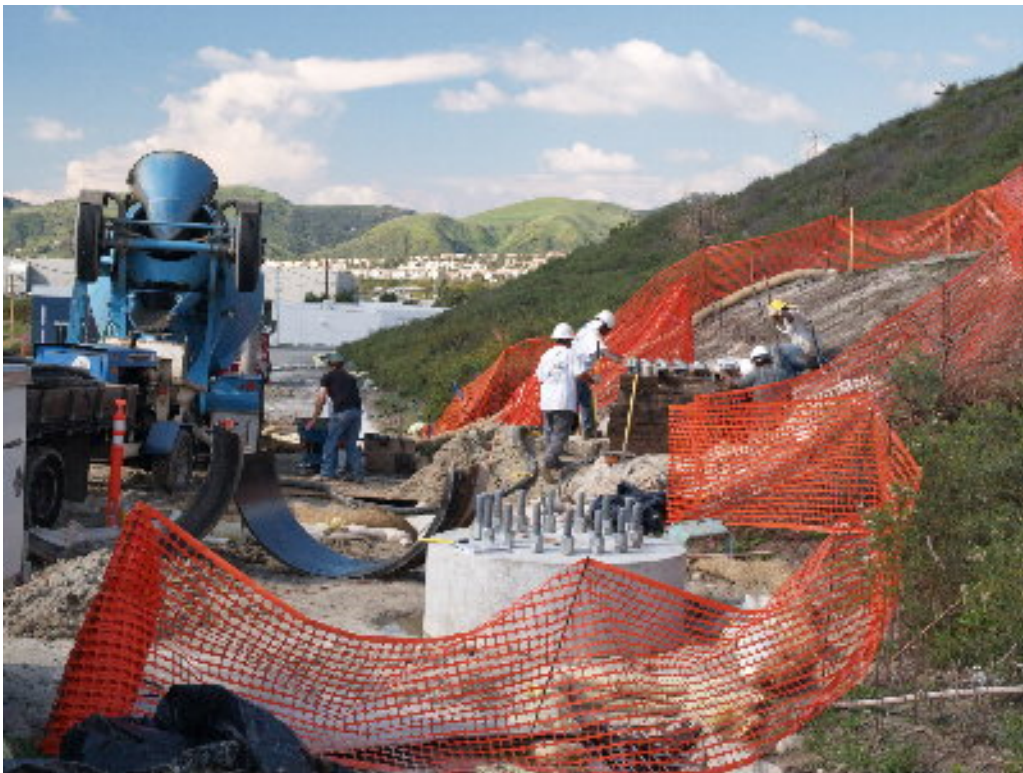
Figure 6 – Inland Valley Construction poured the foundation for the 66 kV steel pole on the edge of the substation site.
