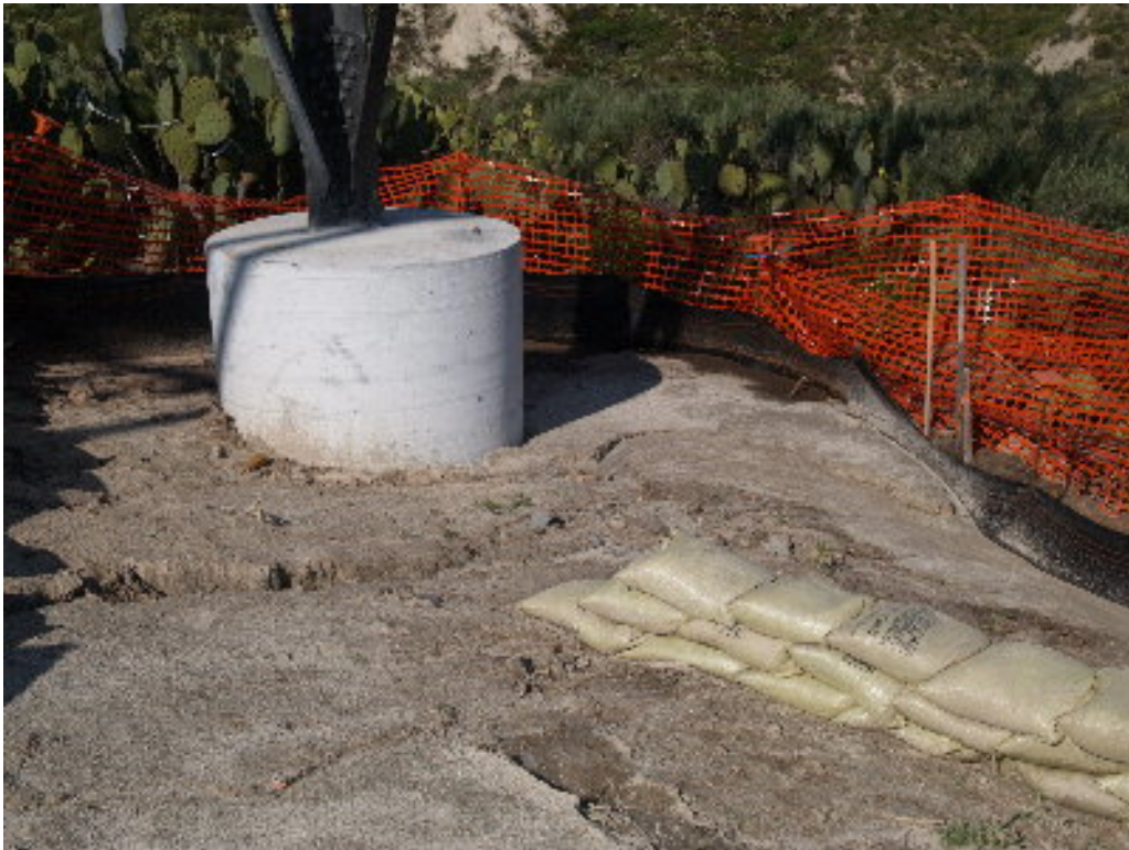
Figure 4 – The silt fencing on the 220 kV transmission line corridor was overwhelmed in several places and still requires maintenance.
