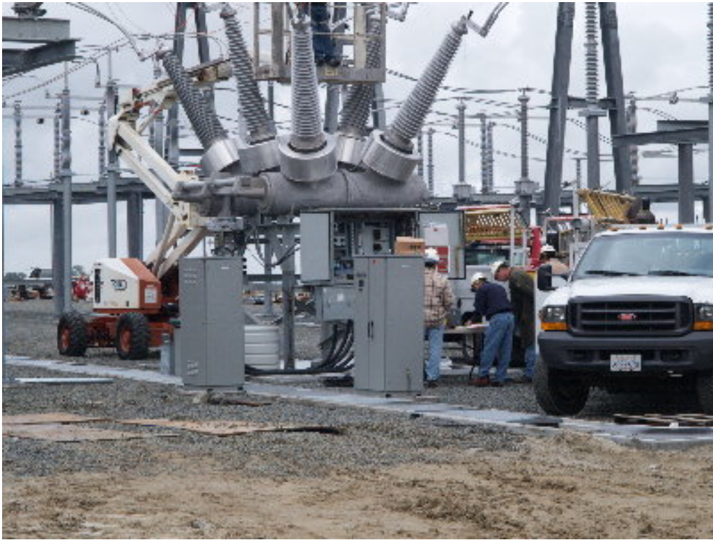
Figure 5 – Crews tested all the panels throughout the substation prior to energizing.
