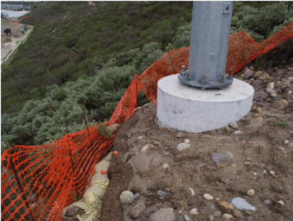
Figure 6 – The BMPs on the pads for the steel poles on the 220 kV section of the project have been overwhelmed and silt has entered the habitat.
