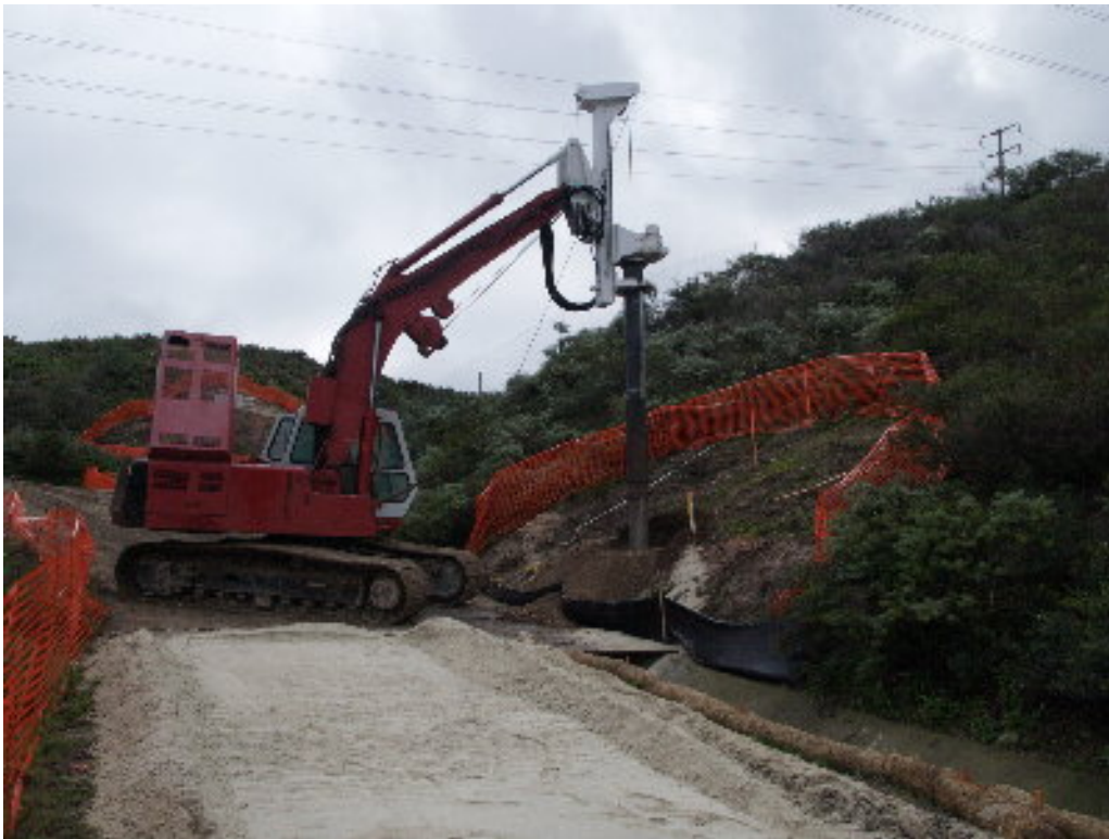
Figure 8 – A Low-Drill was used to work on the final foundation for the 66 kV poles adjacent to the substation site. Drilling spoils will have to be cleaned from the v-ditch.
