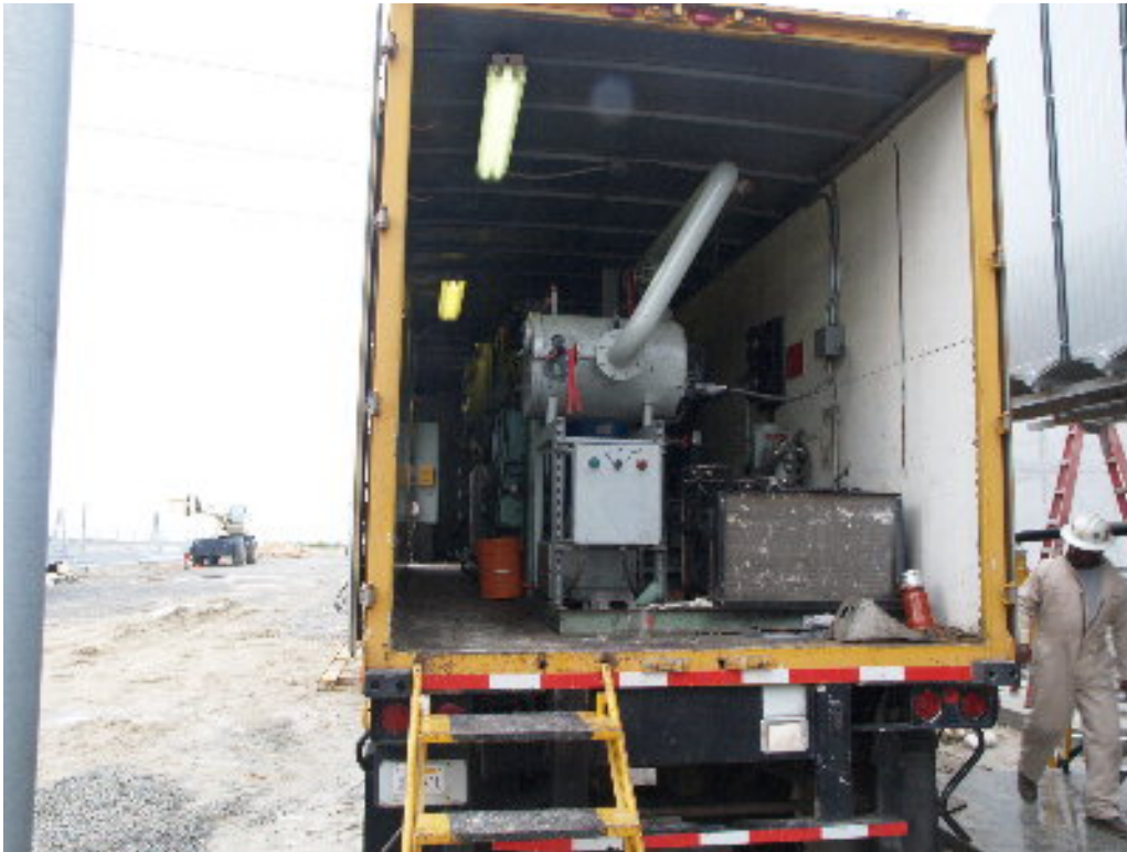
Figure 1 – A SCE crew used a special vacuum to pull the moisture from the A-bank transformers.
