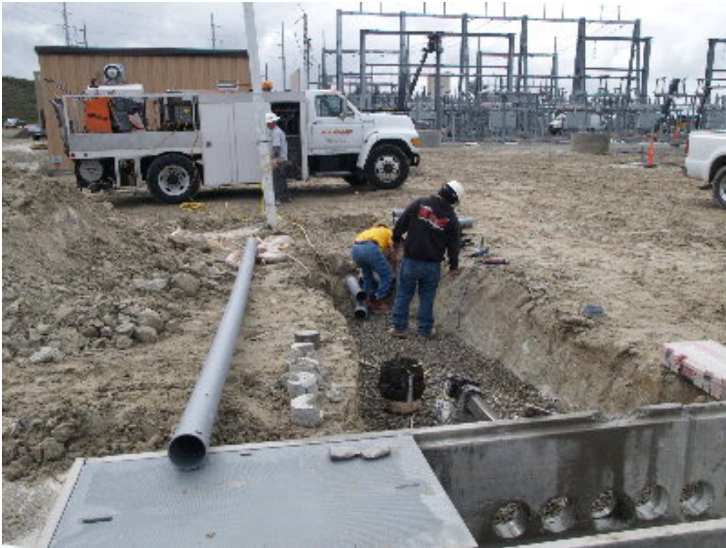
Figure 3 – A crew worked to place conduit for the 12 kV housekeeping power in the prepared trench and into the vault.
