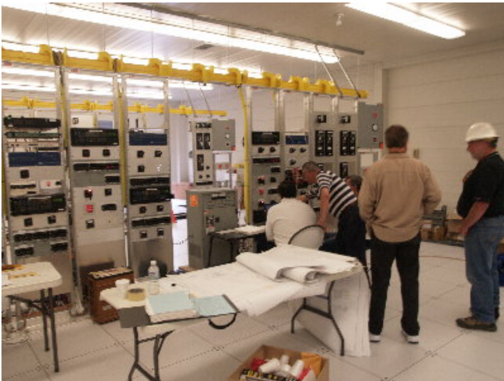
Figure 2 – The control panels in the MEER #1 were tested during the site visit.
