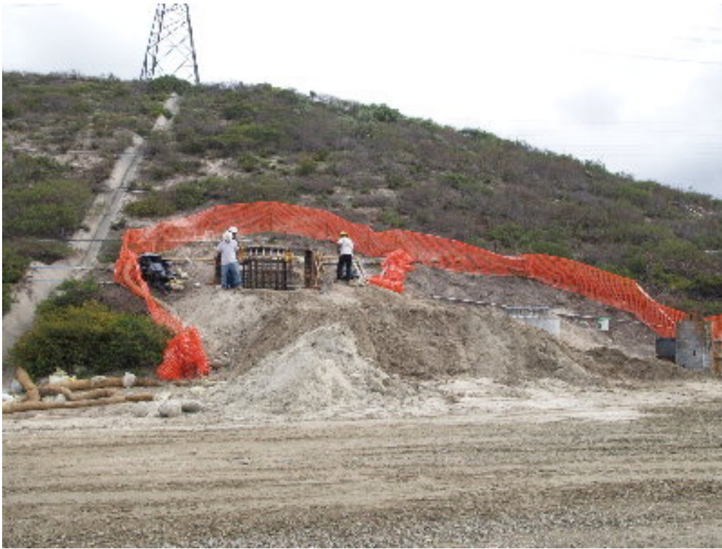
Figure 7 – The Inland crew worked to prepare the second to last foundation for pouring on the 66 kV right-of-way.
