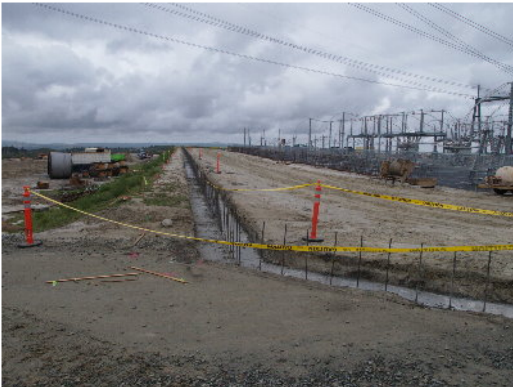
Figure 4 – A Union Construction crew excavated and poured the foundation for the southern portion of the block wall that will surround the substation site.
