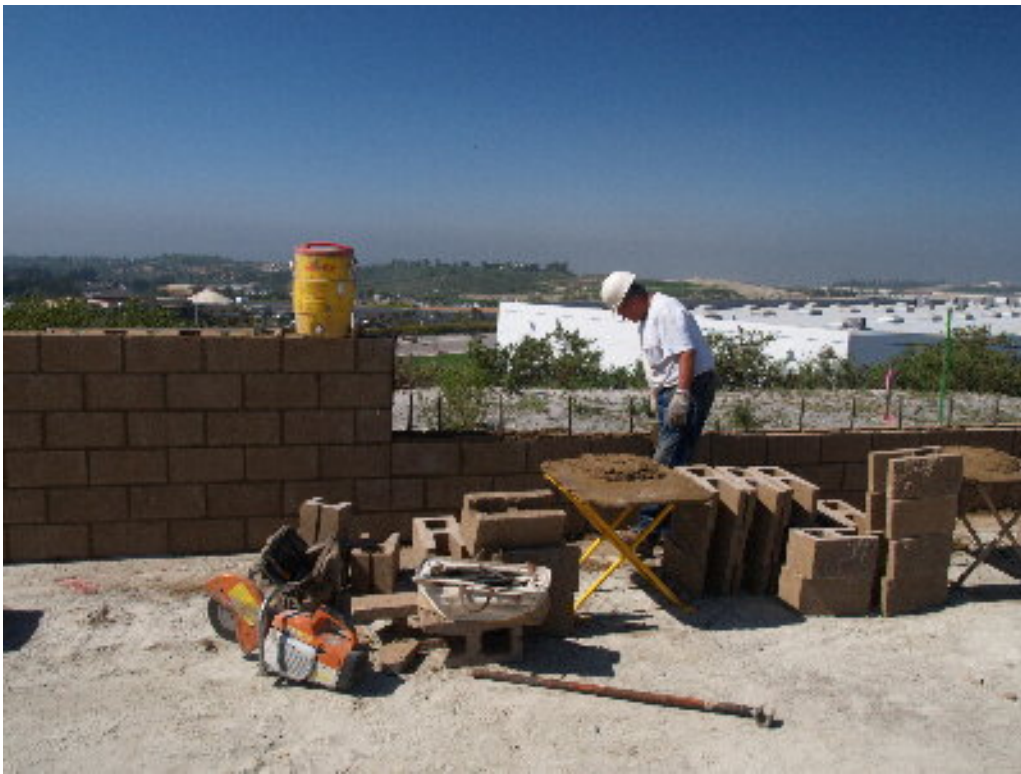
Figure 2 – A specialized crew set the concrete blocks on the west side of the substation during the site visit.
