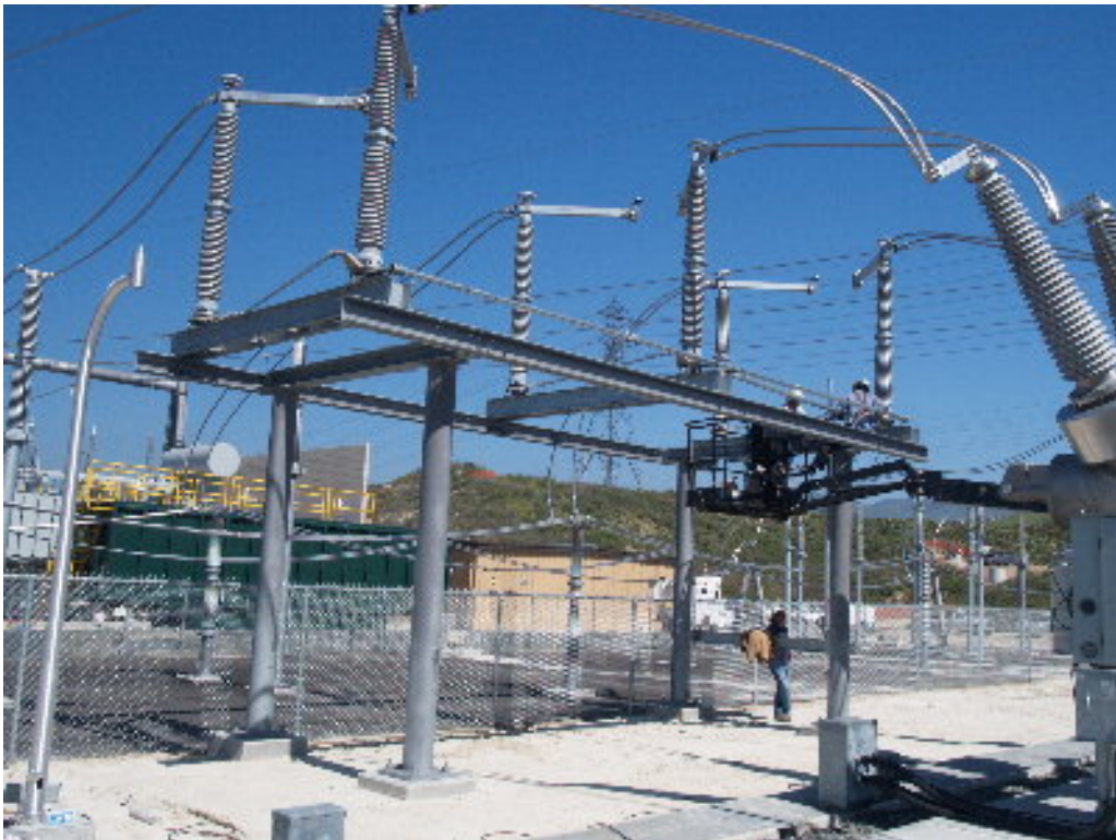
Figure 4 – A small crew worked to adjust the disconnect switches on the 220 kV portion of the substation site.
