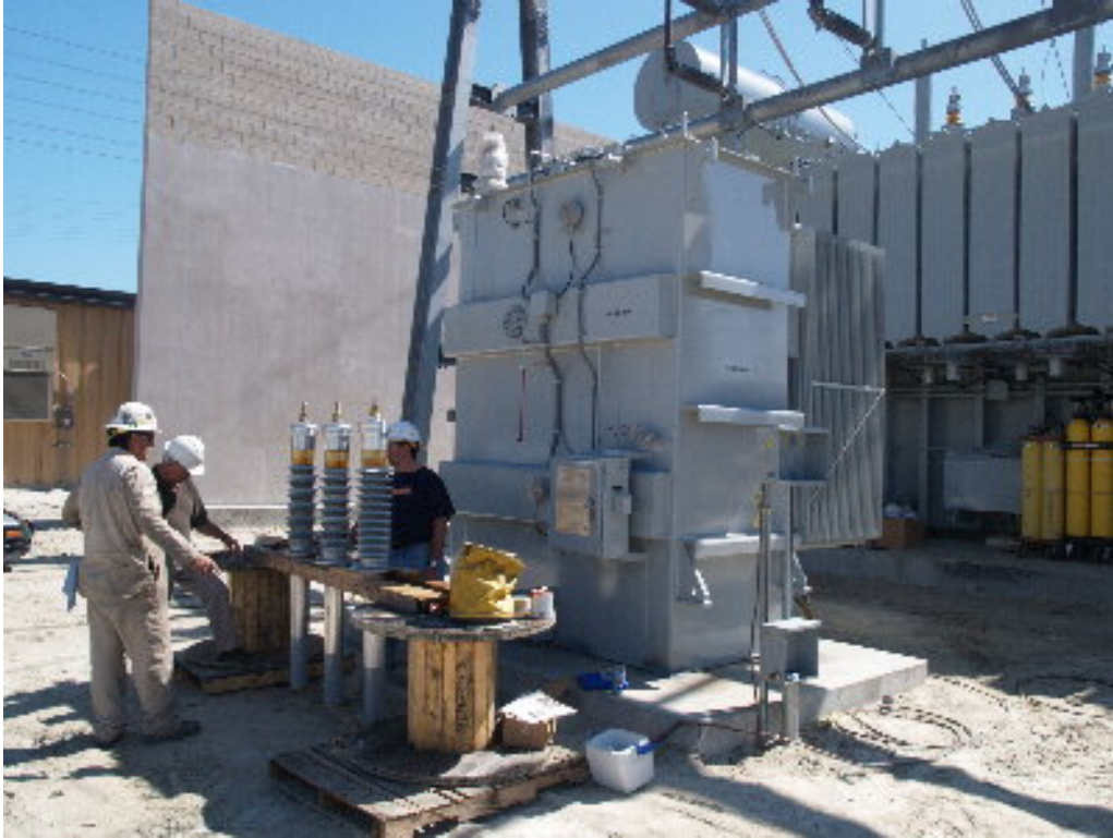
Figure 1 – The grounding transformers for the A-bank transformers have been set on pads and will be connected to the system shortly.
