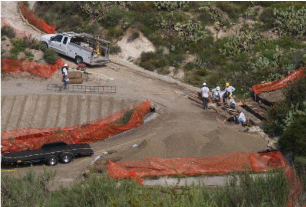
Figure 6 – Crews worked to build forms for the v-ditches on the 66 kV section of the project. Jute netting has been placed on the slopes of the complete steel pole pads.
