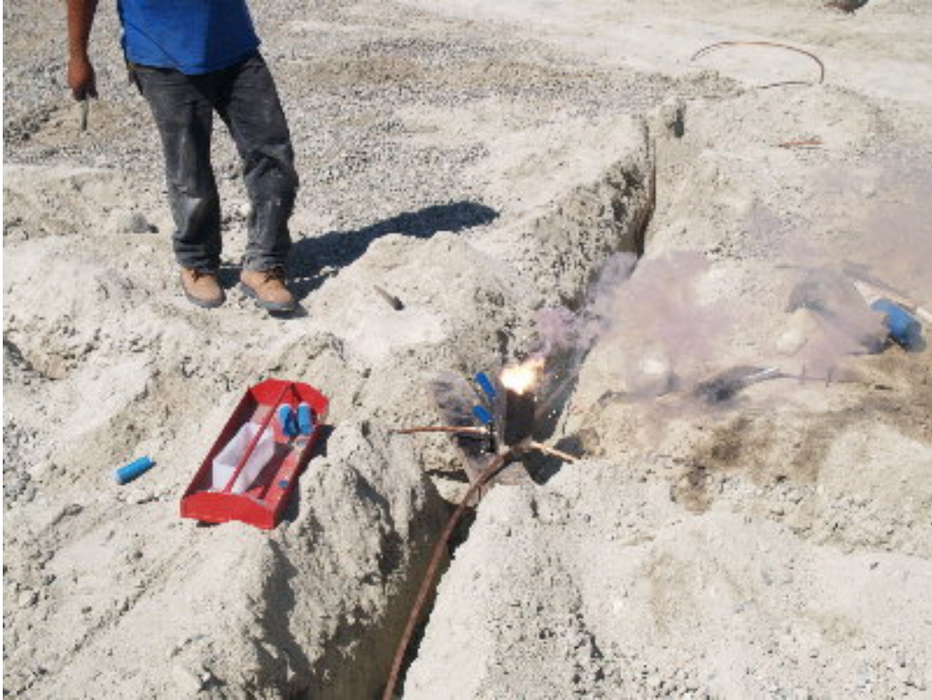
Figure 3 – A small crew worked to fuse connections on the grounding grid that runs throughout the substation site.
