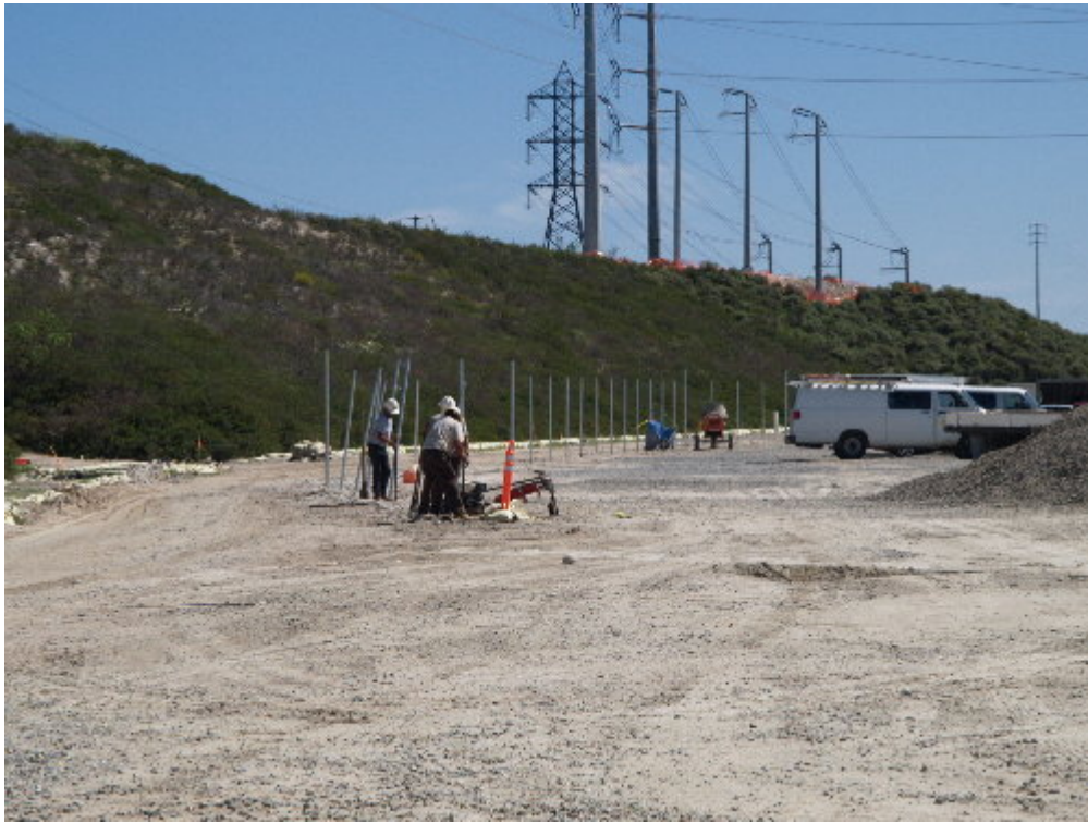
Figure 5 – The poles for the cyclone fence were being set during the site visit. The cyclone fencing will only be on the eastern portion of the substation site and will not be visible from the public right-of-way.
