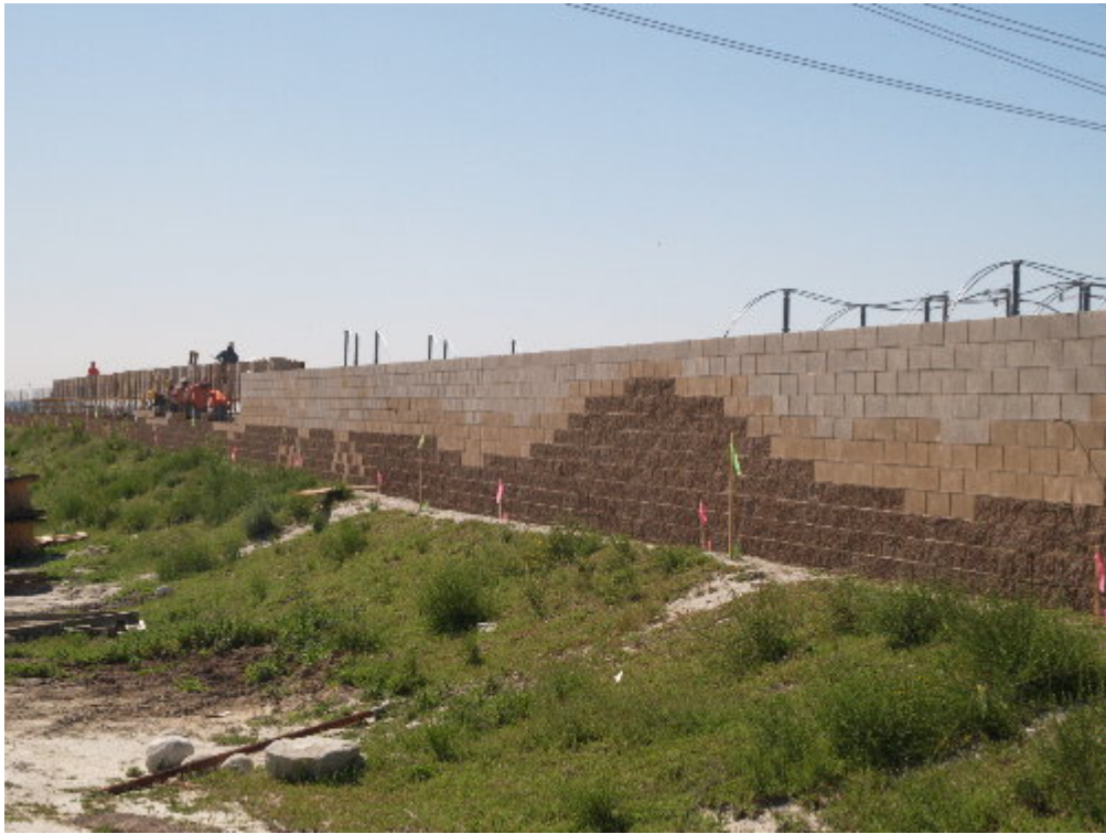
Figure 3 – The pattern of the block wall can be seen now that the upper level has been set. The berm in the foreground will be removed to maintain the required wall height.
