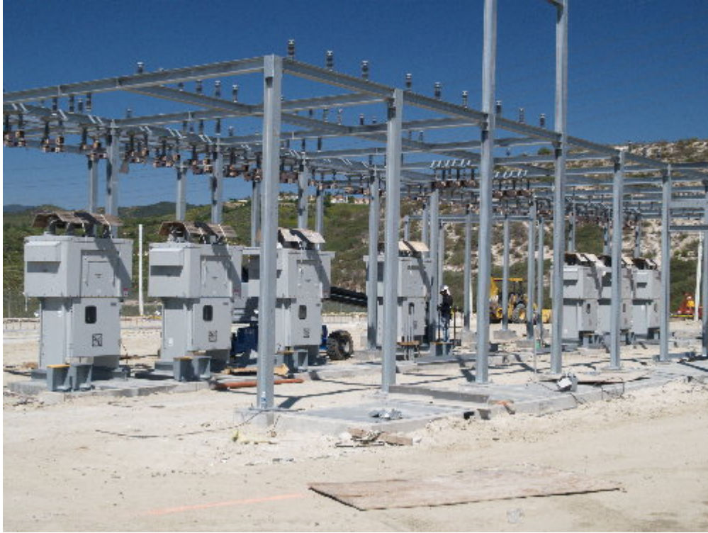
Figure 1 – The disconnects for the 12 kV portion of the substation site have been set.
