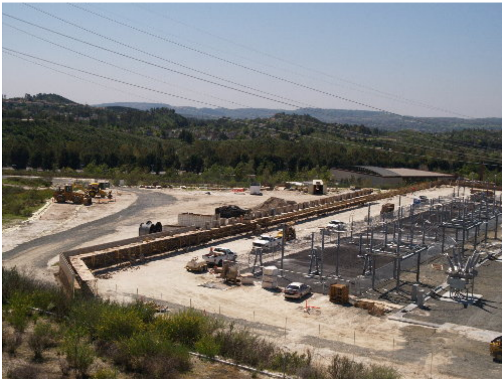
Figure 2 – A specialized crew with Reycon set the upper section of concrete blocks on the south side of the substation during the site visit.
