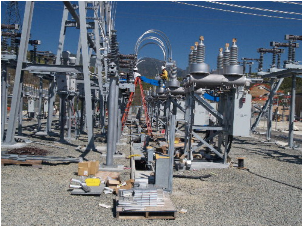
Figure 4 – A small crew with NRG worked on connections on the 66 kV portion of the substation site.
