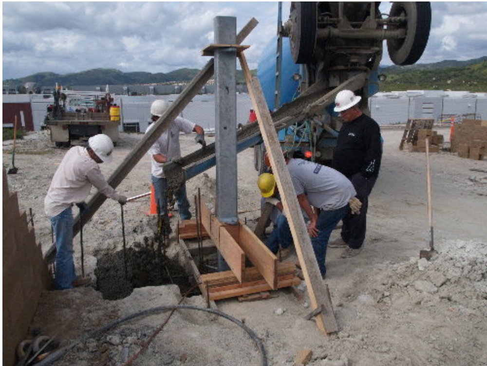
Figure 4 – Union poured the foundations for the main gate posts for the substation site.
