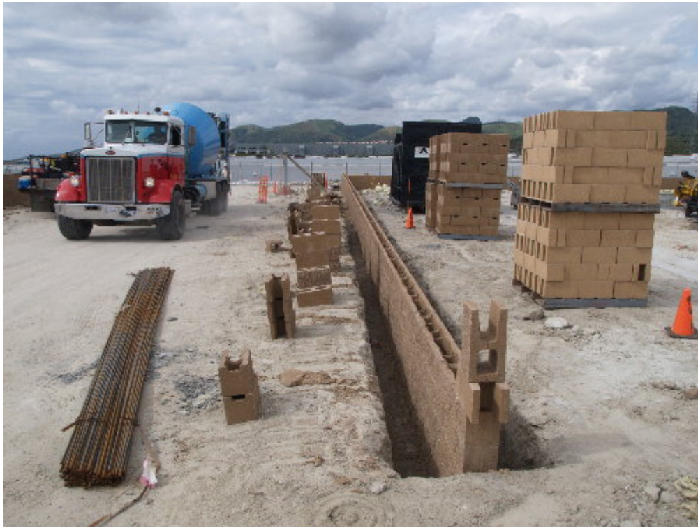
Figure 3 – Reycon started setting the concrete blocks for the spill wall on the north side of the substation site.
