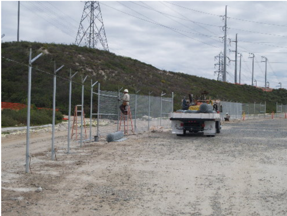
Figure 6 – The fencing was placed on the poles for the cyclone fence during the site visit. The cyclone fencing will only be on the eastern portion of the substation site and will not be visible from the public right-of-way.
