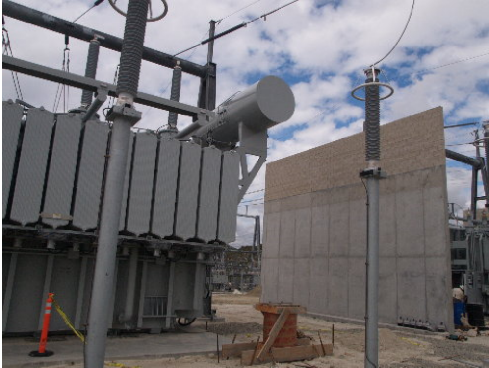
Figure 1 – New poles will be placed to gain the proper off-set between the circuits and the oil tank on the A-bank transformers.
