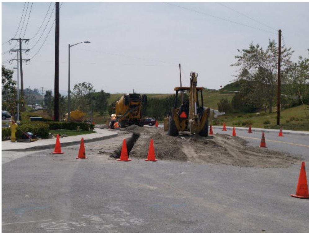
Figure 4 – Arizona Pipeline worked on trenching, laying conduit for the 12 kV distribution conductor, and backfilling with slurry.
