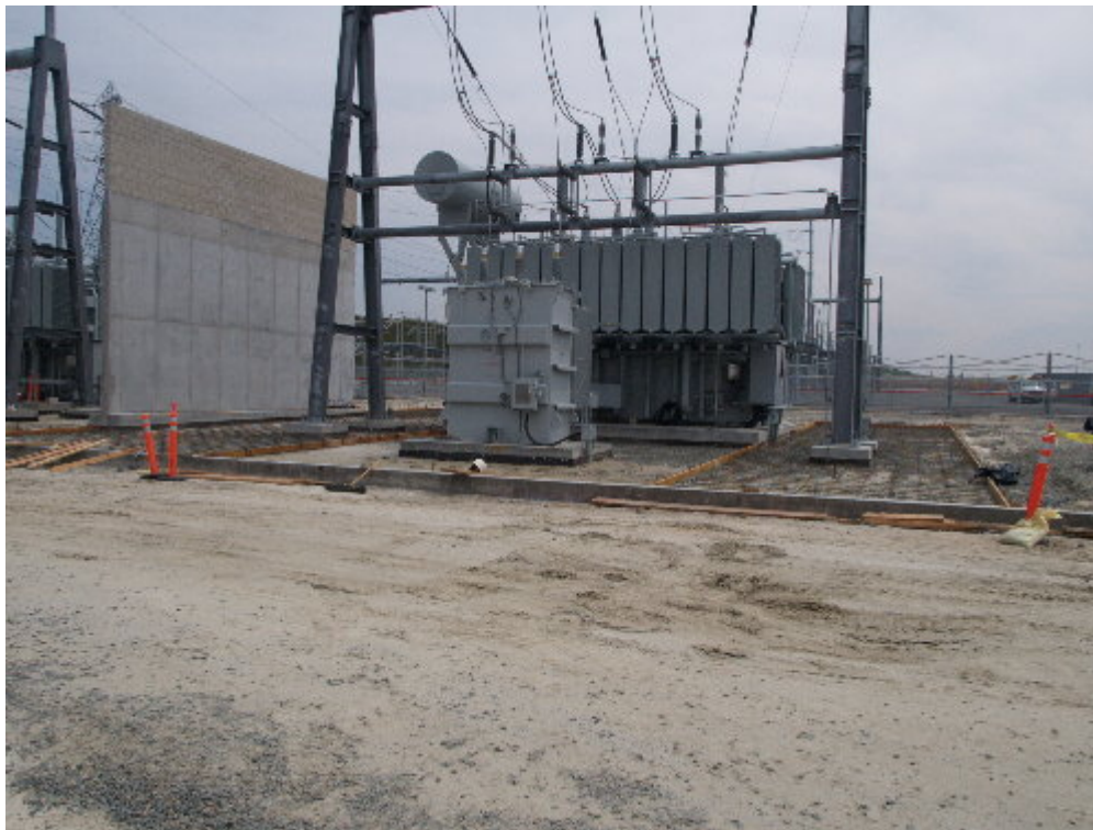
Figure 3 – The forms were set for the concrete pads that will be poured between the various foundations.
