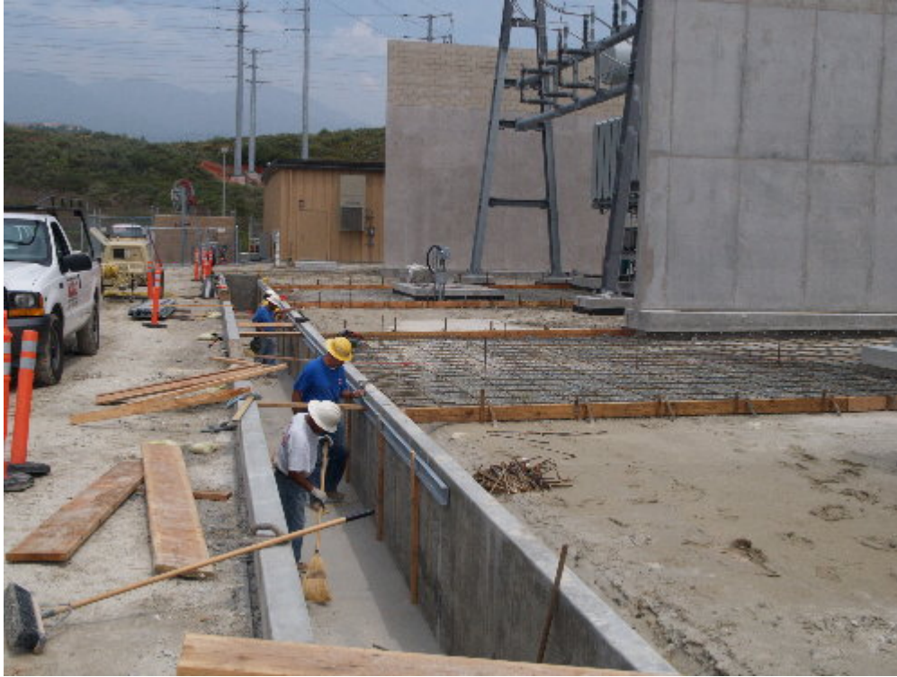
Figure 1 – Crews worked to attach the steel rail that will support the trench covers.
