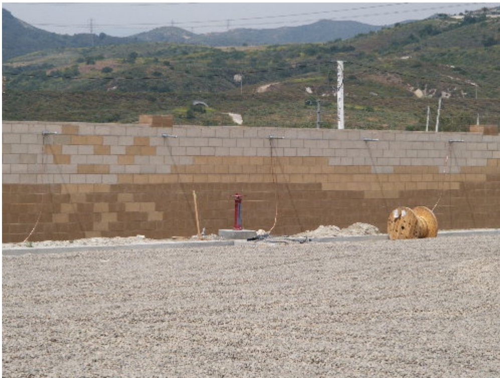
Figure 2 – Reycon worked to ground the barbed wire that runs along the inside of the block wall.
