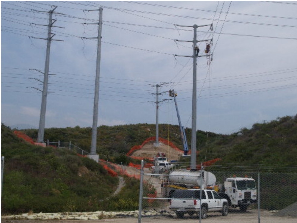
Figure 6 – Crews worked on stringing conductor between the 66 kV line and the substation during the site visit.
