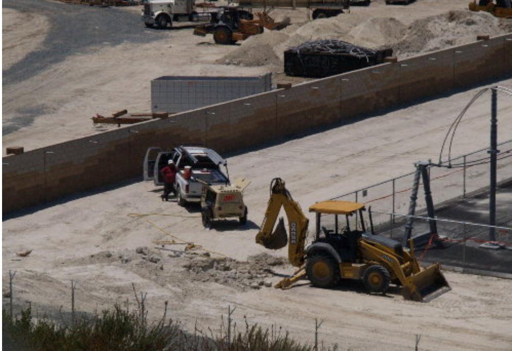
Figure 1 – NRG crews worked on excavating for light standards during the site visit.
