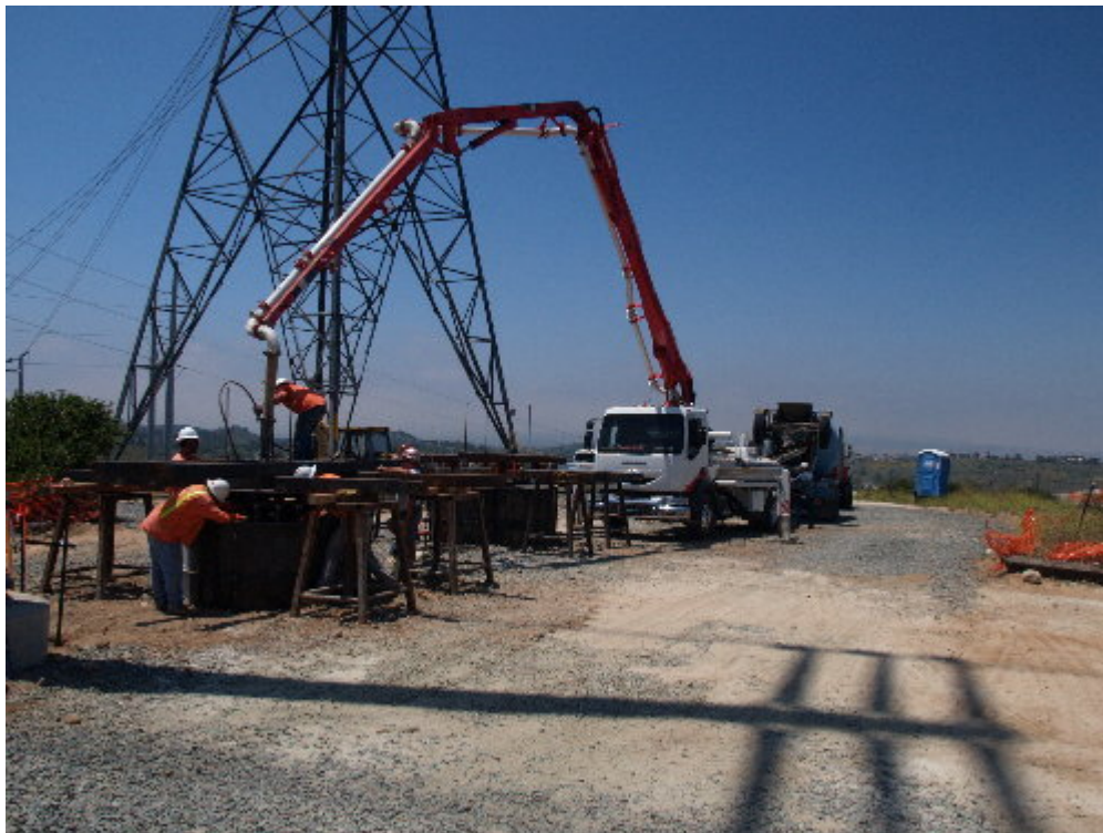
Figure 4 – Arizona Pipeline poured the second foundation for H-Structure 12 during the site visit.
